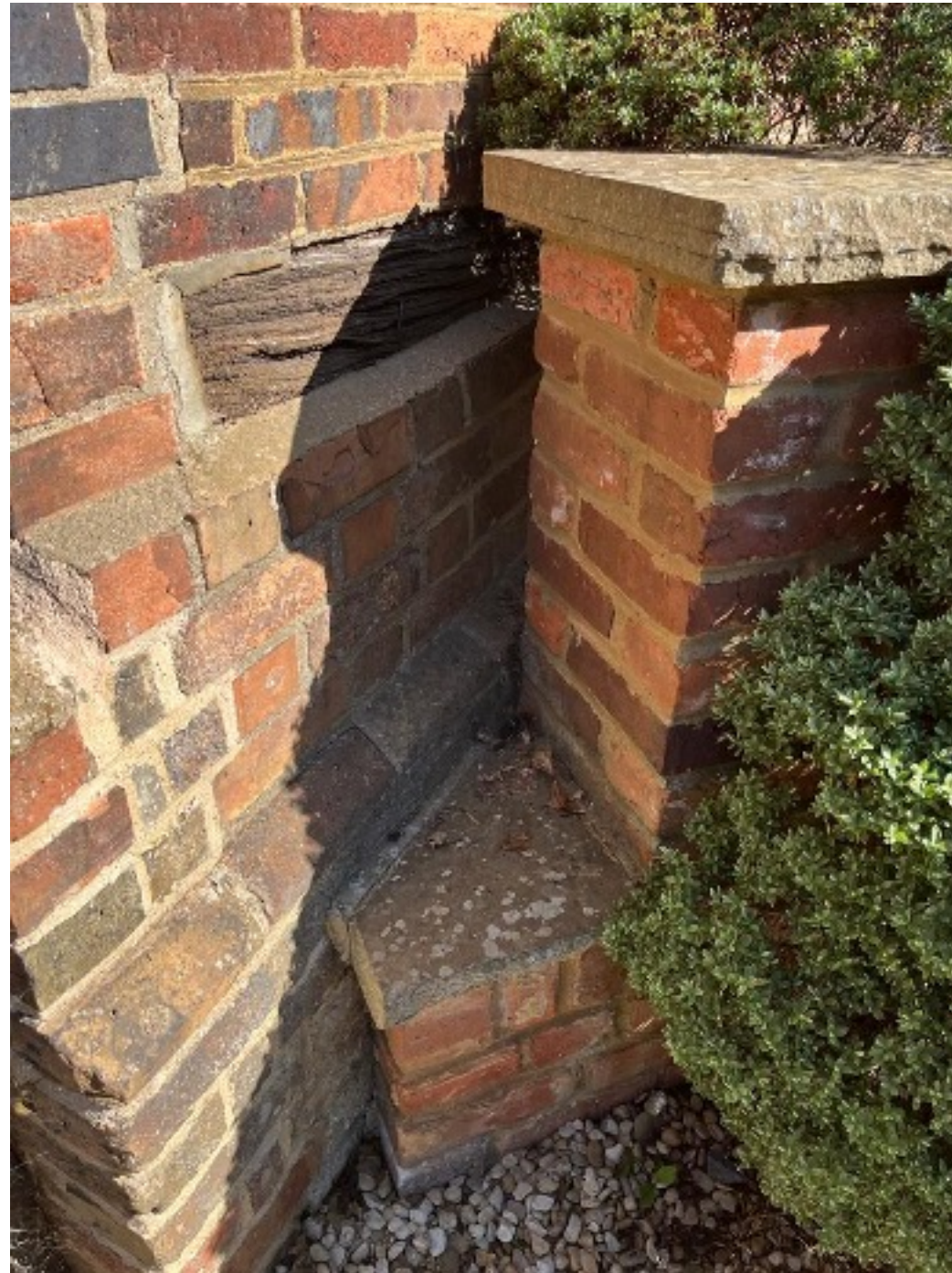
Figure 20: The intersection between the low wall and the house clearly demonstrates that it was a retrospective addition to the property.
