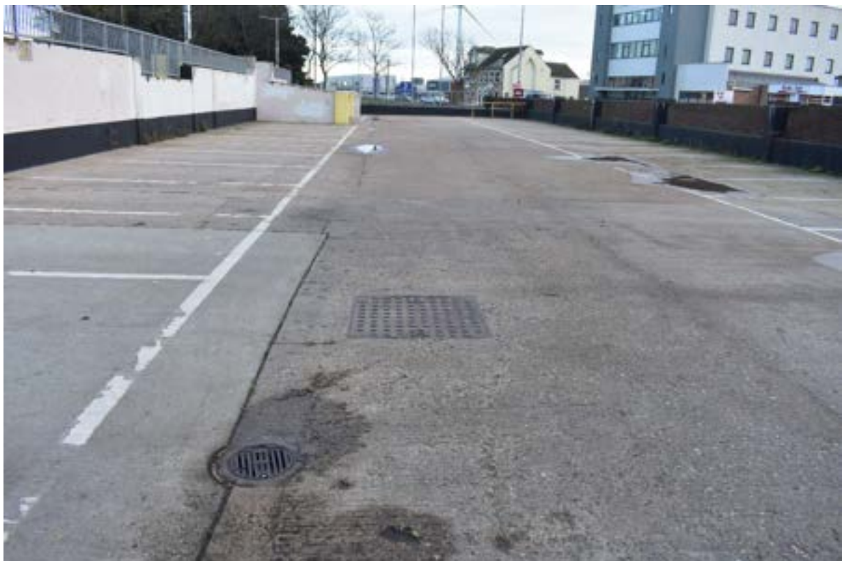
Plate 4: View of the services across the east part of the carpark, looking north-east
