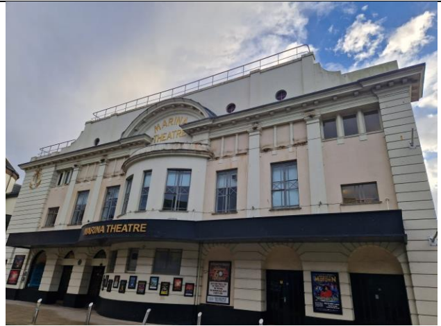
Photograph 6. Main entrance of Marina Theatre with extensive nesting kittiwakes, Avi displacement electric shock system implemented along these ledges.
