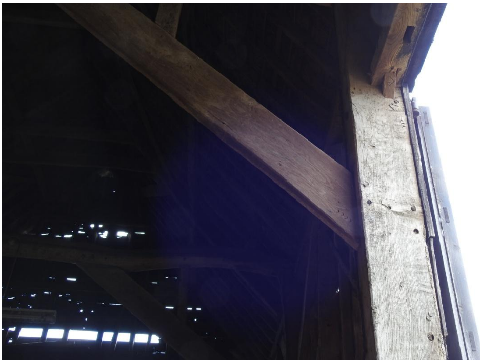
Illus. 12. The eastern storey post of the barn's eastern entrance (1) showing pegs for three mortices in the external face of the timber – two of which bear crescent-shaped carpenter's numerals reflecting that of the tie-beam brace. These mortices are at different heights to those of the rear arcade posts and the rest of the southern posts but match those of the other three door posts –indicating they secured missing porches. Crescent-shaped numbers were cut with a curved race-knife and are not uncommon.
