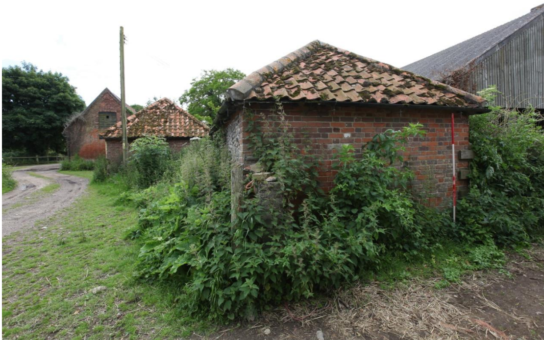
Illus. 22. A detail of the partly rebuilt northern external gable of the small shelter-shed (5) with the cart lodge (3) and cart shed (4) in the rear. The shed's eastern wall consists of flint-rubble with red-brick dressing but the gable has always been of brick. The open-arcade to the west (right) is overgrown and was not fully accessible.
