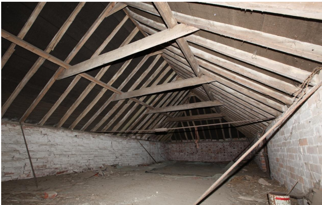
Illus. 18. The undivided hay loft above the stable looking towards its northern gable (2). A number of probably original iron tie-rods span the walls and secure the roof-plates to the floor joists in the absence of tie-beams. The clasped-purlin roof structure consists of uniformly sawn softwood with a ridge-board and nailed collars in the manner of the mid-19 th century.
