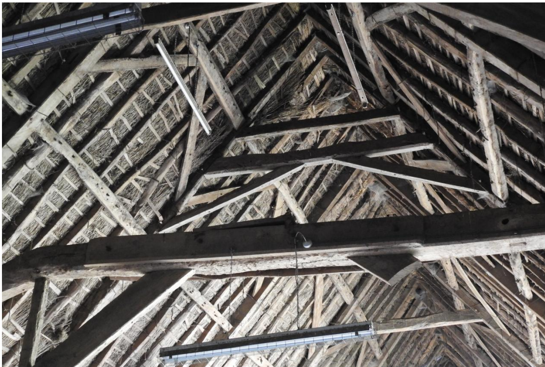
Illus. 14. The unique double collared truss in the centre of the roof with medieval-style diagonal soulaces to the chamfered lower collar. The roof is otherwise typical of the mid-17 th century but the principal rafters are stepped for clasped rather than butt-purlins and the purlins themselves contain irrelevant peg and nail holes indicating re-use.
