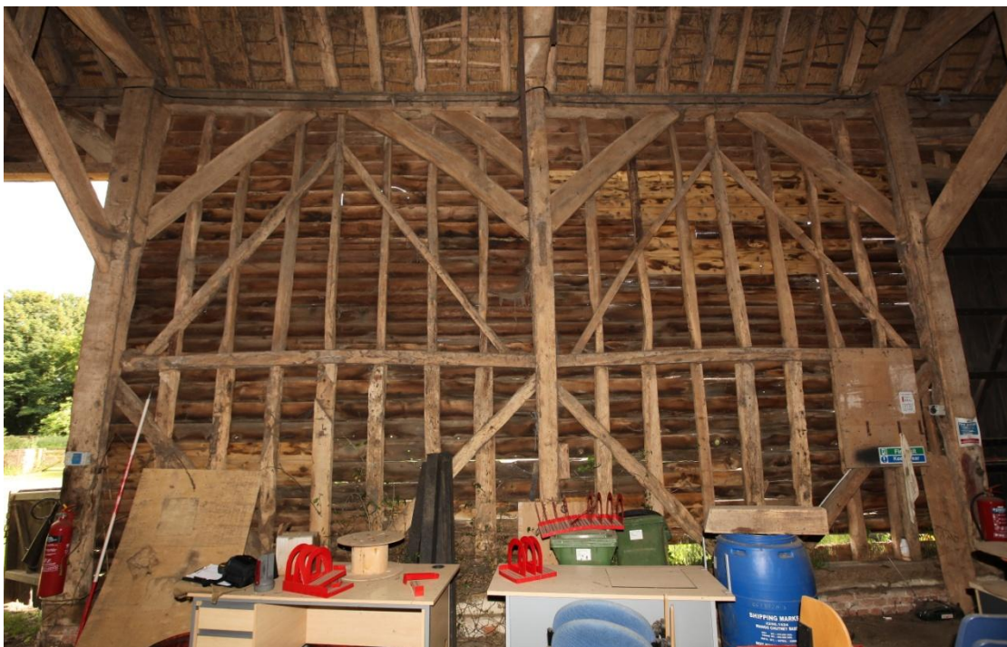
Illus. 10. The central bays of the barn's southern wall (1) showing the arcade braces of a missing front aisle. The framing beneath consists of mid-rails and vertical studs cut by diagonal primary braces all nailed in place in the style of the 19 th century. Note the unique inner brace to the left of the central post, possibly designed to support a scarf.
