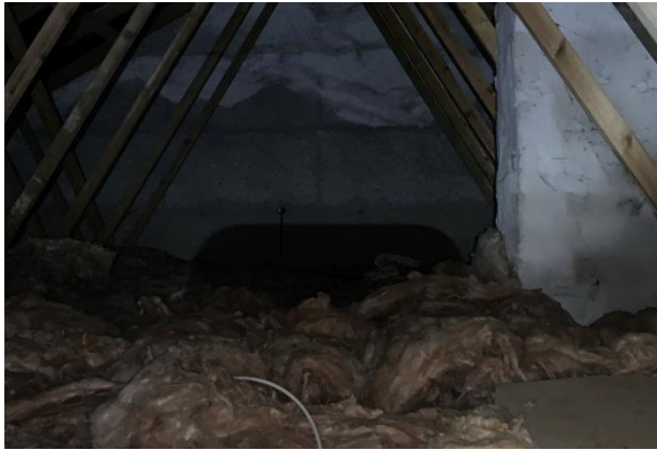
Photograph 3: Example of void insulation, fibre glass wool insulation buildings B1 – B11.
