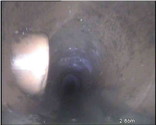
MH40X_b2c4e567-22d3-473a-81bf-3acf1dde1ad3_20231009_115330_022.jpg, 00:00:12, 2.86 m Connection defective, connecting pipe is intruding at 9 o'clock, 150mm dia, intrusion: 15%
