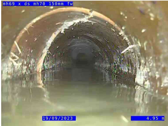
MH69X_d9ec47a4-55a2-49e9-aba4-c6384b44d033_20231009_143550_266.jpg, 00:00:31, 4.95 m Broken pipe at joint from 9 o'clock to 1 o'clock
