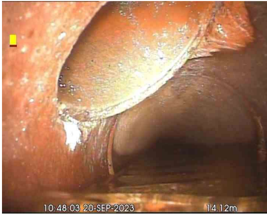
MH73X_22f6e67d-f3a7-48f1-b0f6-ed899fecf2e7_20231009_150523_113.jpg, 00:01:14, 14.12 m Connection defective, connecting pipe is intruding at 10 o'clock, 100mm dia, intrusion: 10%
