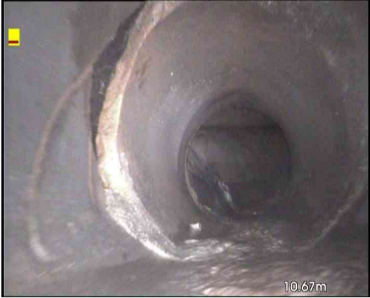
MH111X_24ed393f-d370-4503-8dd2-ed27a5e1a155_20231010_130829_433.jpg, 00:00:39, 10.67 m Hole in drain or sewer from 8 o'clock to 11 o'clock, AT JOINT
