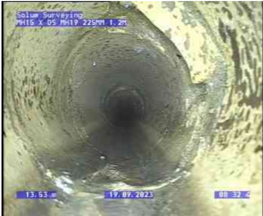
MH15X_d63fadcb-f4bc-4ce1-bf2c-d67bd93a6ca3_20231005_093226_393.jpg, 00:01:33, 13.53 m Connection defective, connecting pipe is intruding at 2 o'clock, 150mm dia, intrusion: 10%
