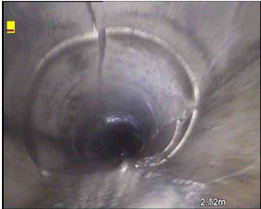
MH109X_4b2bd999-5c50-4281-97c5-ff718d8d337c_20231010_124514_836.jpg, 00:00:08, 2.52 m Broken pipe from 12 o'clock to 12 o'clock, start
