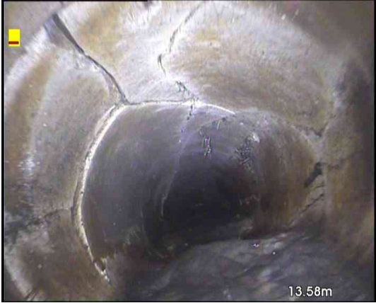
MH85X_aad4b9dc-b431-400a-b544-8d6517d1163e_20231010_085405_737.jpg, 00:00:44, 13.58 m Broken pipe from 12 o'clock to 12 o'clock, start
