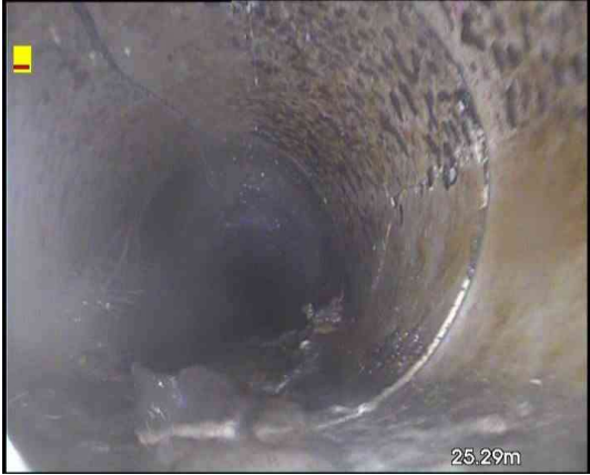
MH92X_33d811c1-21be-4341-8c1e-9bb512064dab_20231010_093544_866.jpg, 00:01:06, 25.29 m Broken pipe at joint from 5 o'clock to 7 o'clock
