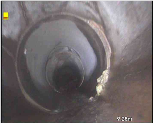
MH100X_45827f3d-dbab-42b7-94f4-a32c2b7531d5_20231010_105807_665.jpg, 00:00:28, 9.28 m Broken pipe at joint from 1 o'clock to 3 o'clock
