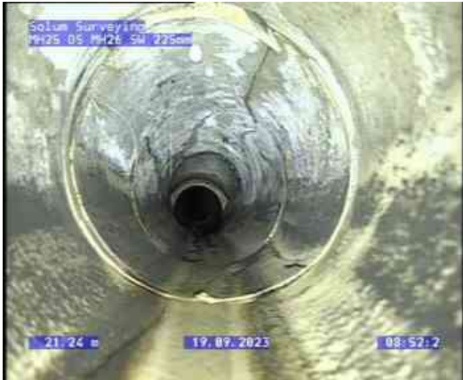
MH25X_8f274589-b94c-46e7-b1d7-ca2fcd8f8a65_20231005_132932_738.jpg, 00:01:38, 21.24 m Broken pipe at joint from 11 o'clock to 2 o'clock
