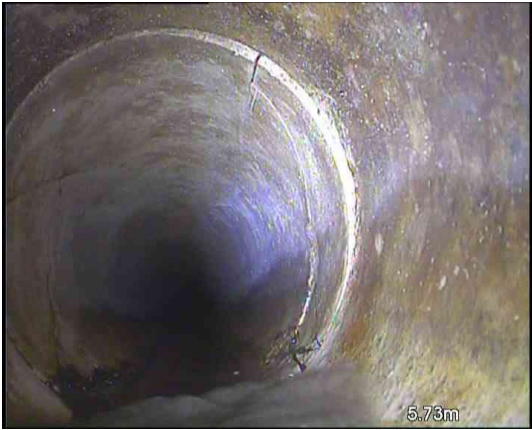
MH28X_a1b8e47f-44b9-4217-b8c7-c67eff98a3eb_20231005_140825_157.jpg, 00:00:26, 5.73 m Broken pipe at joint from 1 o'clock to 5 o'clock
