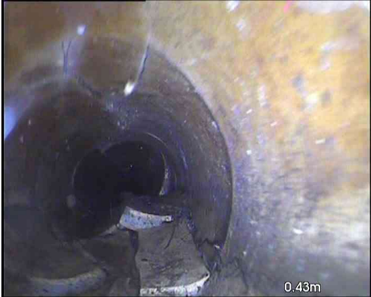
MH18X_588d93d8-0691-423b-9591-348c62ca6498_20231005_095307_681.jpg, 00:00:09, 0.43 m Broken pipe from 12 o'clock to 12 o'clock, start
