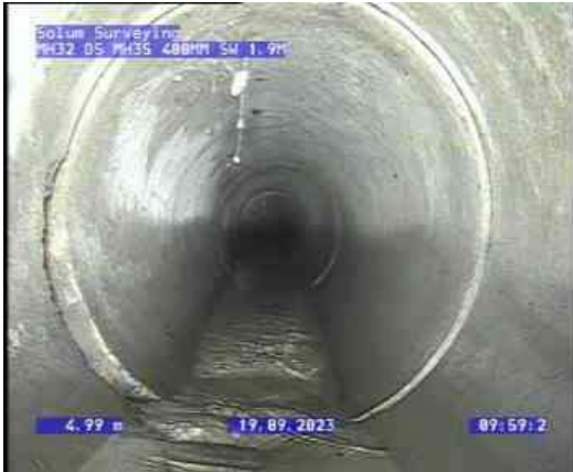
MH32X_bb127f40-8b4d-4311-a8cb-ed932acd47ee_20231009_112338_379.jpg, 00:00:32, 4.99 m Broken pipe at joint from 7 o'clock to 9 o'clock
