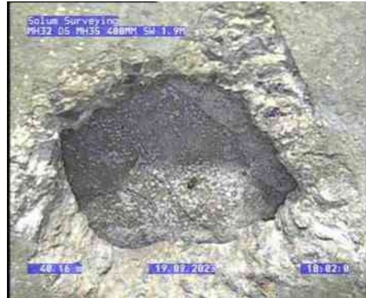
MH32X_38f532f4-52d5-430e-b97b-07a4197883f7_20231009_112625_027.jpg, 00:03:06, 40.16 m Hole in drain or sewer at 12 o'clock
