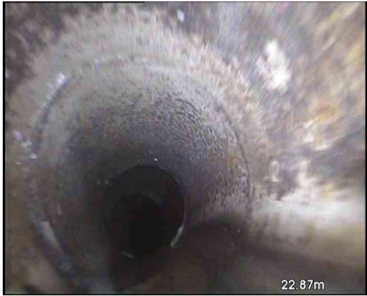
MH4X_6a5e938b-03c7-4156-a8c1-0e94677db67a_20231004_150639_924.jpg, 00:01:04, 22.87 m Broken pipe at joint from 7 o'clock to 9 o'clock
