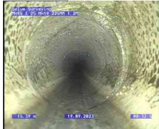
MH15X_416a6b17-5e09-4cf9-8eb4-2279ff69c08e_20231005_093340_645.jpg, 00:01:44, 15.39 m Broken pipe at joint from 11 o'clock to 2 o'clock
