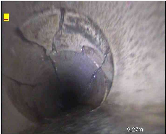
MH110X_89f44c82-90f9-47f9-b718-c8fdcbcd1237_20231010_130203_874.jpg, 00:00:22, 9.27 m Broken pipe at joint from 11 o'clock to 3 o'clock
