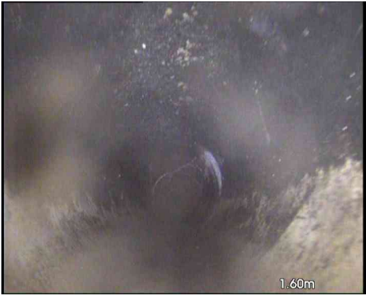
MH6X_7f79ca1b-f459-435c-90fc-8602aeb7b4ea_20231004_1 51019_865.jpg, 00:00:11, 1.28 m Broken pipe at joint from 4 o'clock to 7 o'clock
