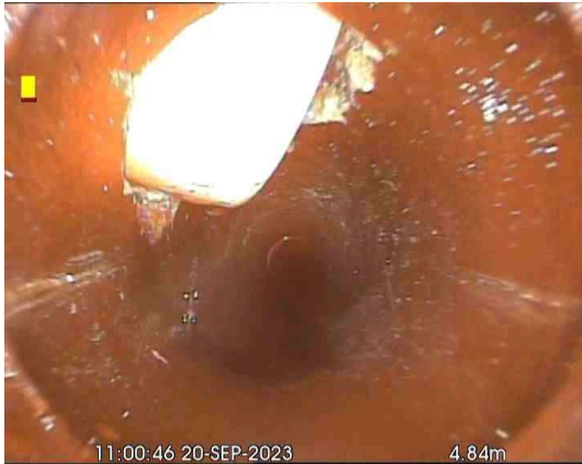
MH76X_39ae886e-d3eb-443a-ac5e-132a0f62dc9e_20231009_153203_374.jpg, 00:00:21, 4.84 m Connection defective, connecting pipe is intruding at 10 o'clock, 100mm dia, intrusion: 10%
