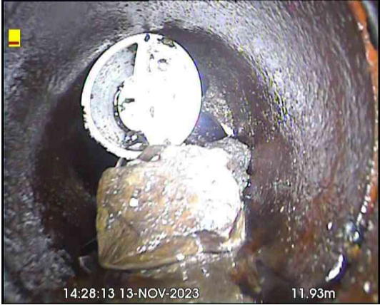
USX_01b41d0b-e175-4bf8-9f72-47c53c03f0bb_20231129_075333_931.jpg, 00:00:48, 12.28 m Settled deposits, other, 90% cross-sectional area loss
