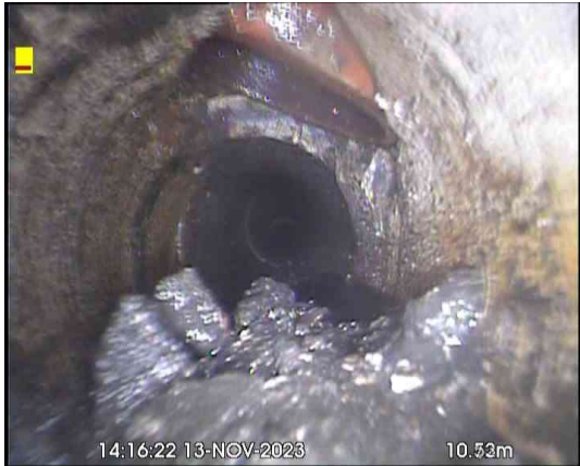
USX_f2865516-4e09-4abd-a0f9-6cf901975f0f_20231129_080052_211.jpg, 00:00:53, 10.53 m Connection defective, connecting pipe is damaged at 1 o'clock, 100mm dia
