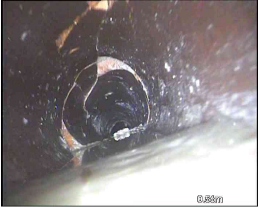
MH27X_db4a563b-b4b5-4986-9509-74b73bd5f2af_20231005_134650_419.jpg, 00:00:08, 0.56 m Broken pipe from 9 o'clock to 3 o'clock, start
