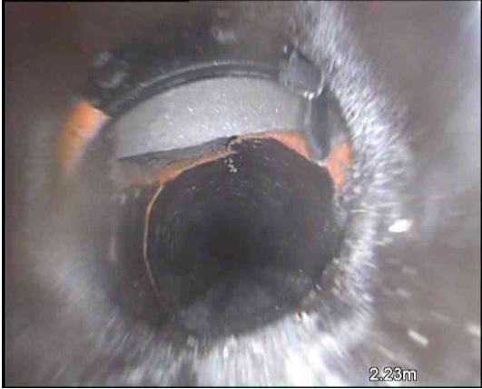
MH16X_6743155c-b319-4636-a4e1-6ab9b0ba6bbe_20231005_092050_334.jpg, 00:00:15, 2.29 m General remark, POSSIBLE HOLE OR CONNECTION AT 12 O CLOCK
