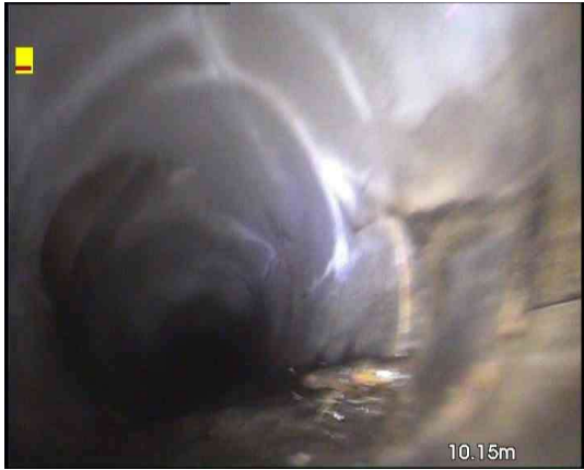
MH103X_fc04fbc2-a940-4b29-af7a-296cc7654755_20231010_114540_106.jpg, 00:00:29, 10.15 m Broken pipe from 3 o'clock to 5 o'clock
