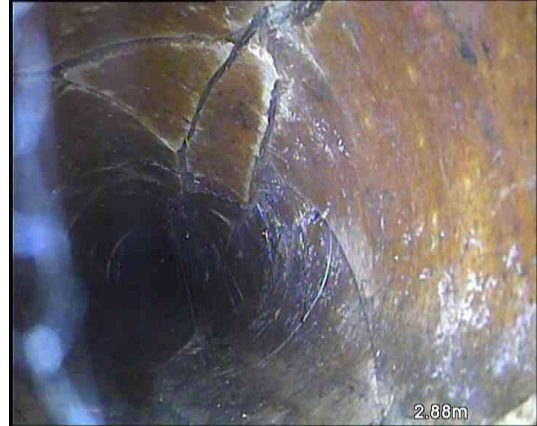
MH18X_51db5a45-6395-4f44-8e17-cb4a92bb53c2_20231005_095448_313.jpg, 00:00:21, 2.89 m Broken pipe from 12 o'clock to 12 o'clock, start
