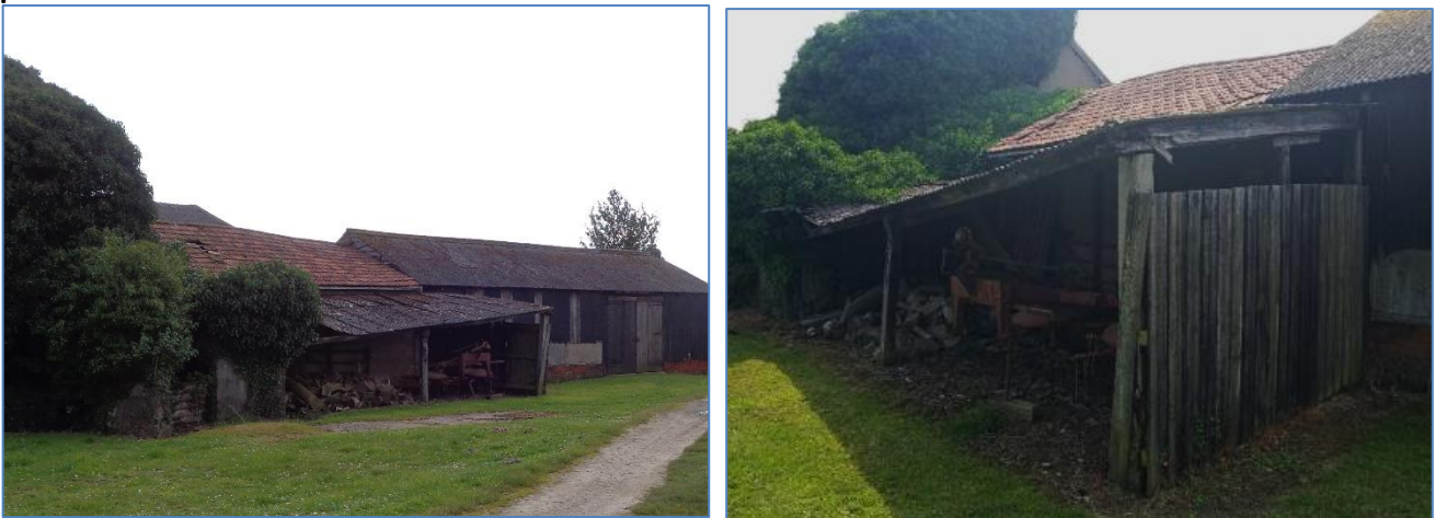
Barn 3 with the collapsed lean to at the rear and Barn 4 in the background, the cartlodge lean to partly collapsed in front of this
