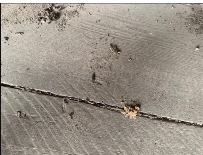
c) B1, bat dropping found on stairs.
