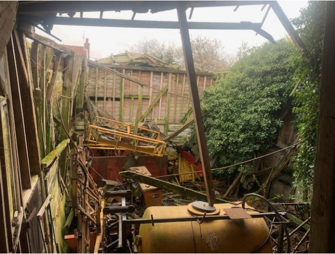
d) Eastern aspect with collapsed roof.
