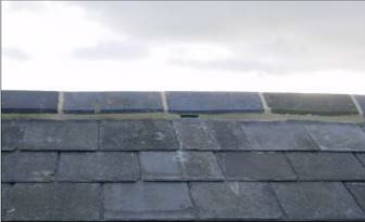
a) Gap beneath ridge tile of slate roof.
