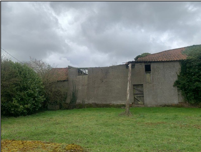
b) Northern aspect showing missing roof.
