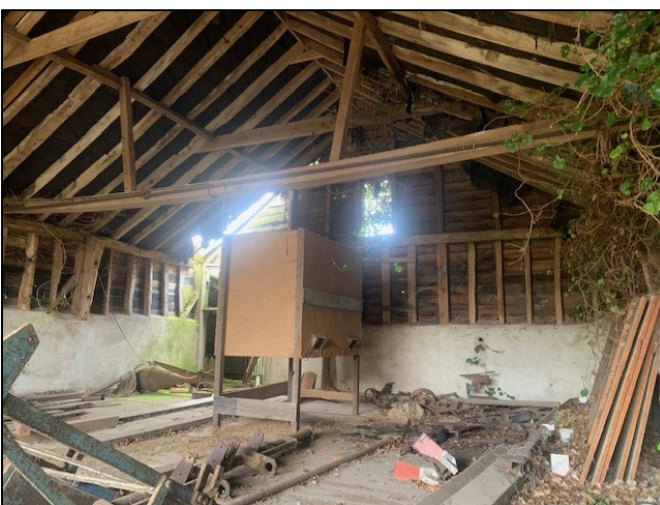
c) B1, mezzanine level. Scattered bat droppings found on the floor.
