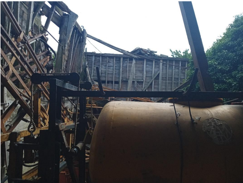
Fig 9. Threshing Barn 1. East bays, roof collapsed and softwood studs visible.
