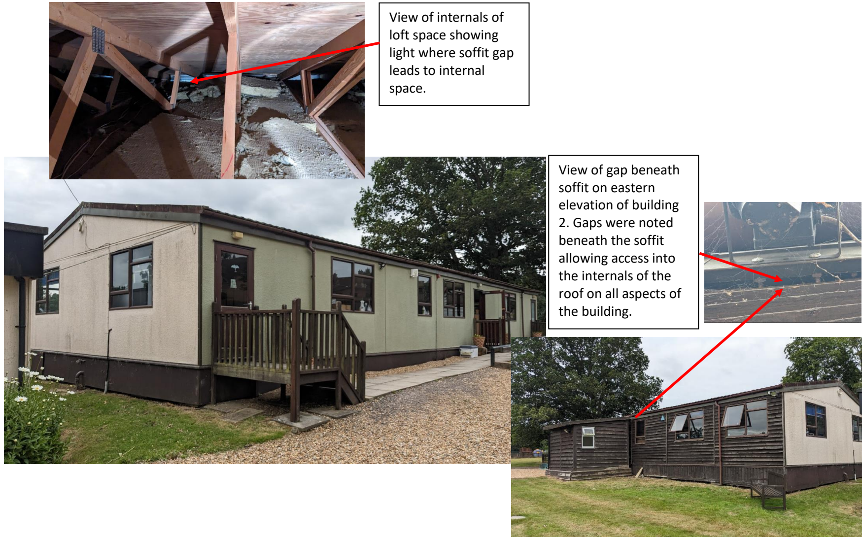
Figure 6. View of western elevation of building 2 and supporting images of PRFs and eastern elevation (taken July 2023).
