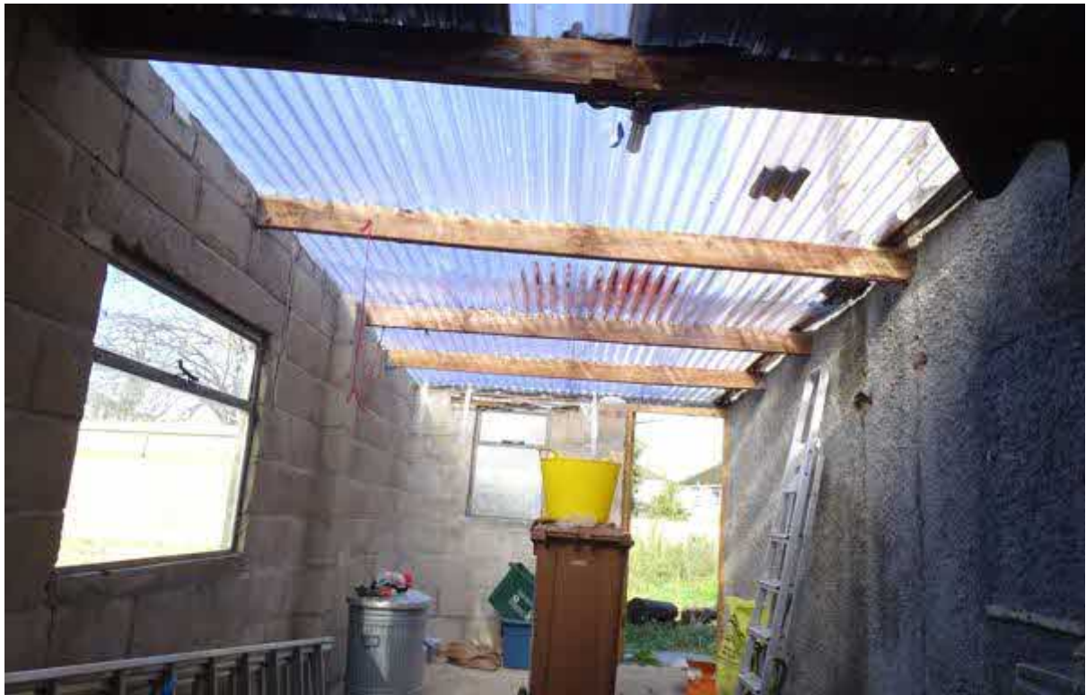
Image 7 – Internal view from within the garage section of the property which has demonstrated a clear fabricated sheet roof covering
