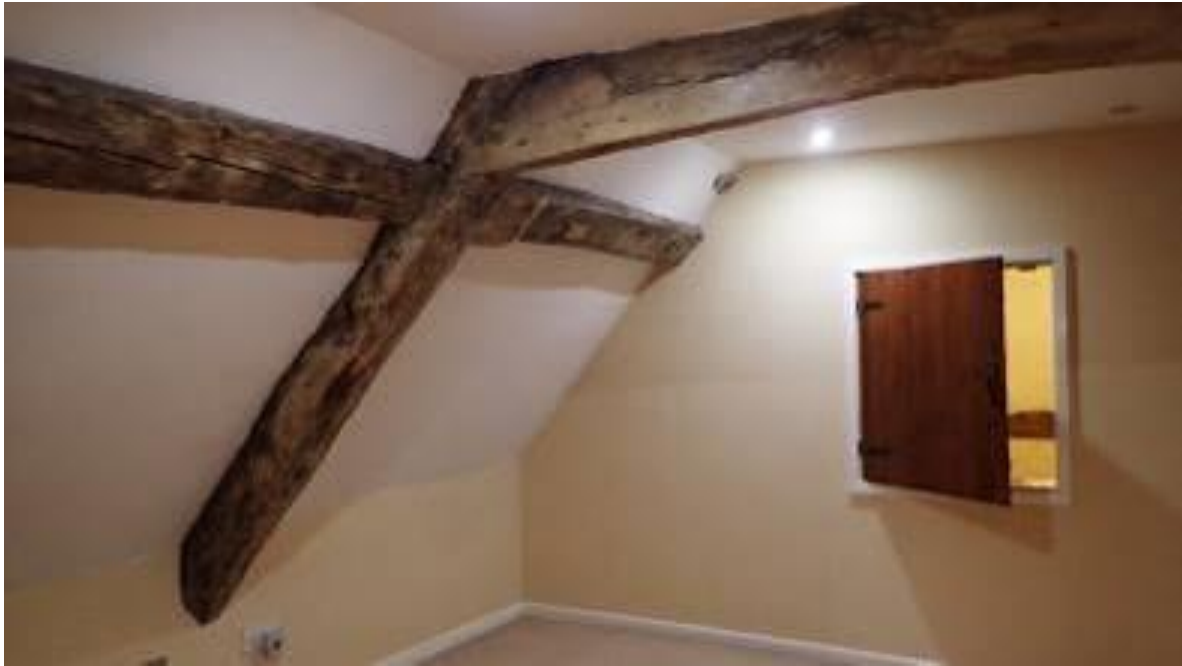
Photograph 4: Interior of first floor room of west section of house showing purlin and tie beam of roofing frame
