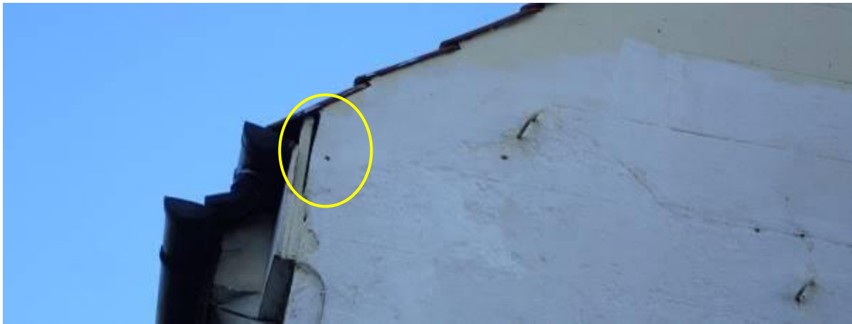
Photograph 12: Gap behind barge board at west elevation of house
