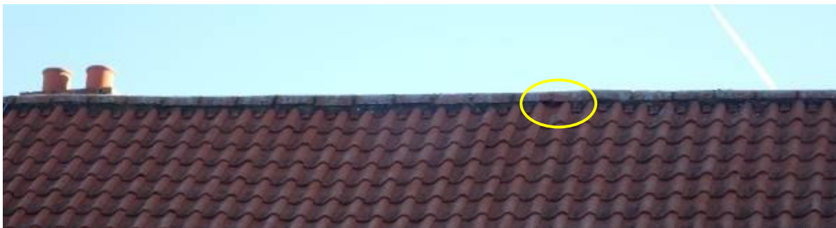
Photograph 10: Gap in beneath ridge tile at west aspect of house
