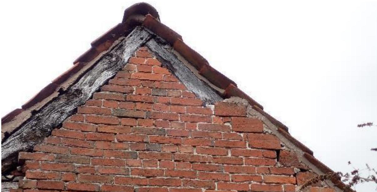
Photograph 15: East gable of outbuilding including gaps around timber roofing frame and in brickwork
