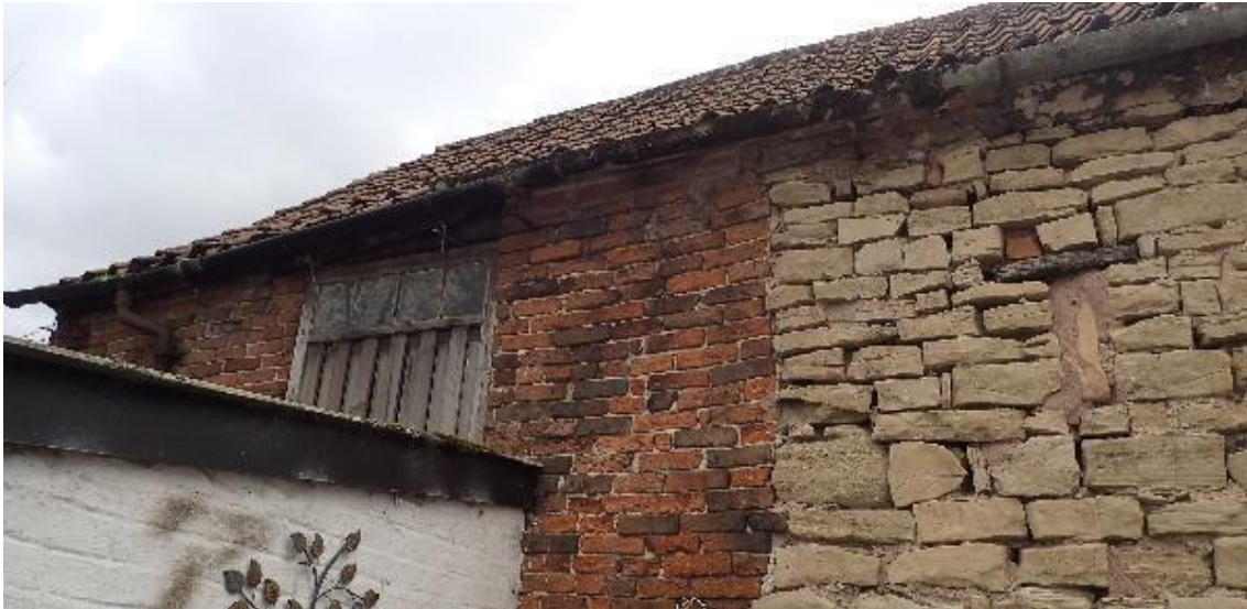
Photograph 16: North elevation of outbuilding with gaps in stonework
