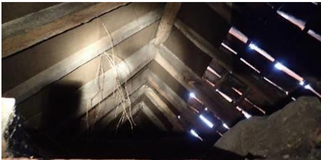
Photograph 13: Roof void of outbuilding showing gaps between pantiles and bitumen felt liner
