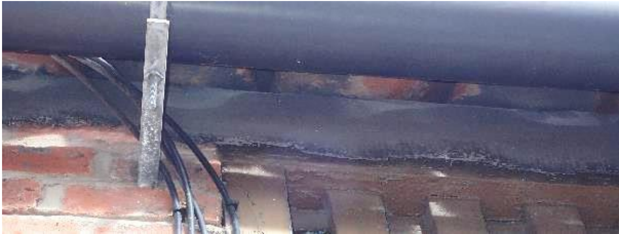
Photograph 14: Overhang of bitumen felt liner at south elevation of outbuilding
