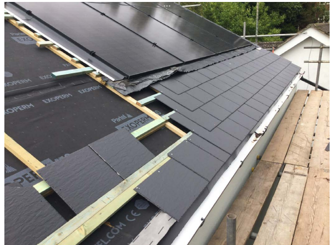
Slate roof with integrated PV panels to rear slope
