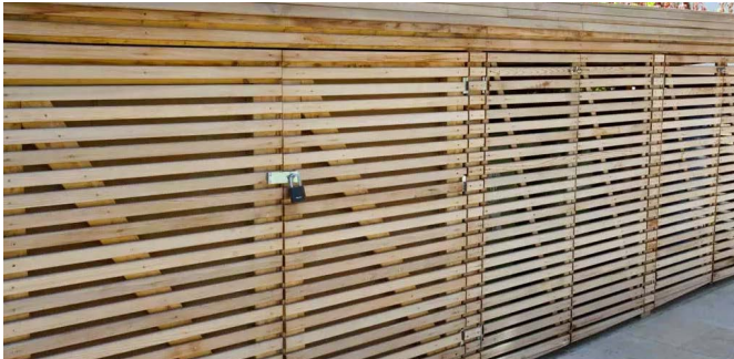
Timber bin store (ventilated)
