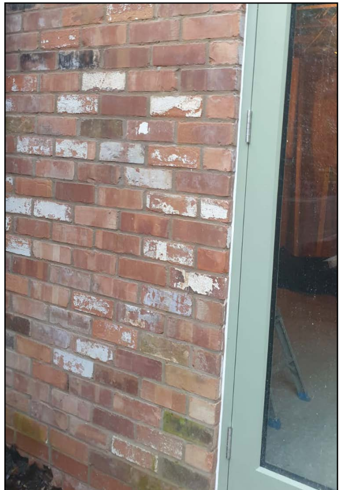
Brick wall to rear facade (bricks reused from demolished structures from site)
