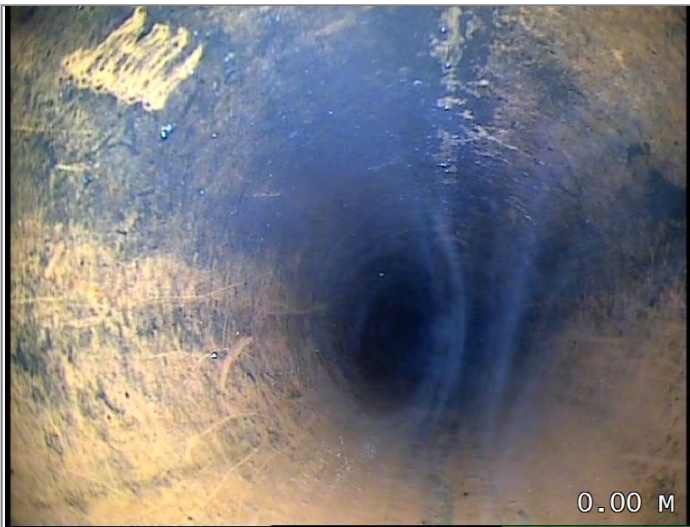
Start node type, inspection chamber, reference MH9
