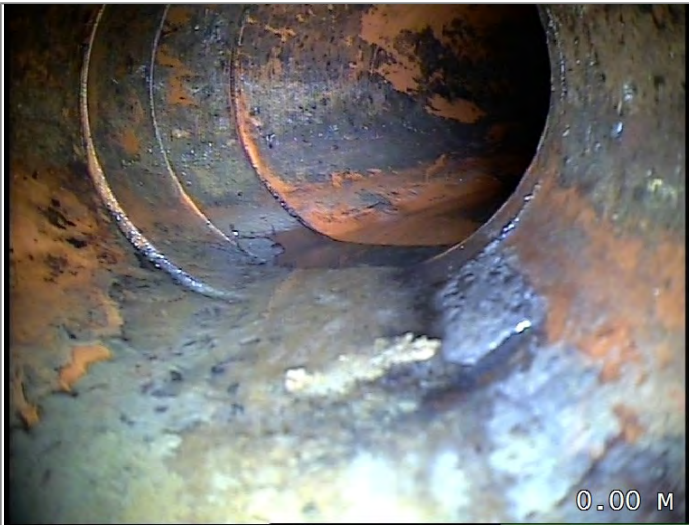
Start node type, inspection chamber, reference MH6
