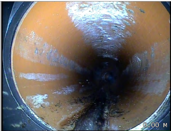
Start node type, inspection chamber, reference MH5
