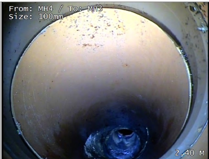
Line of drain/sewer deviates down
