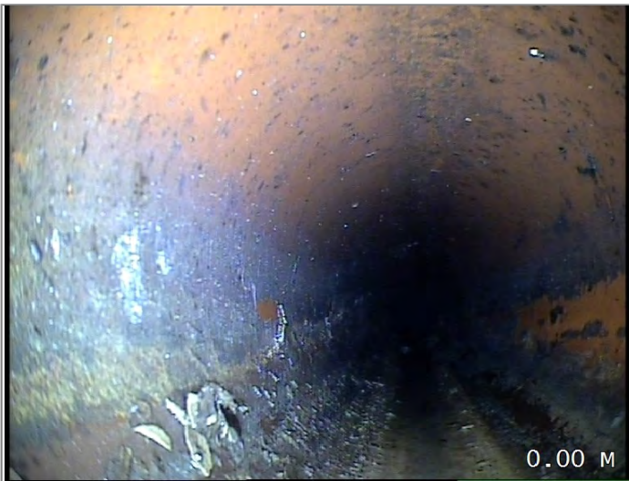
Start node type, inspection chamber, reference MH6
