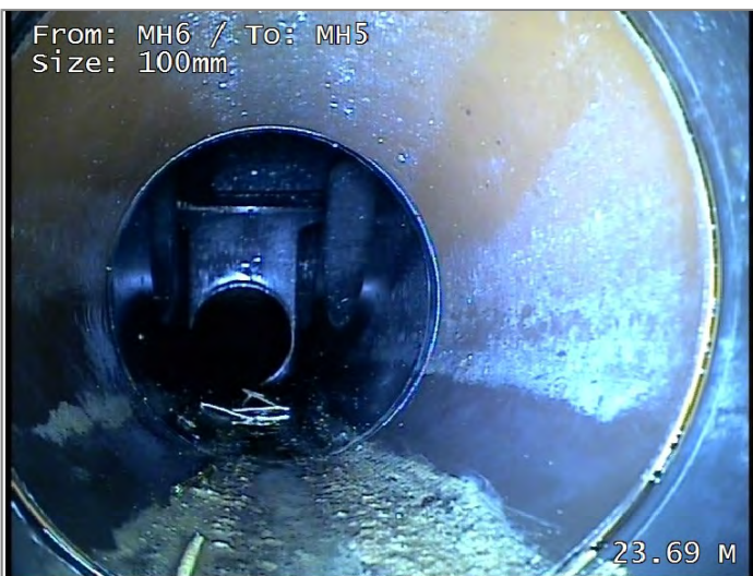
Line of drain/sewer deviates left
