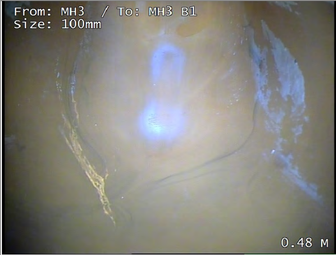
Line of drain/sewer deviates up
