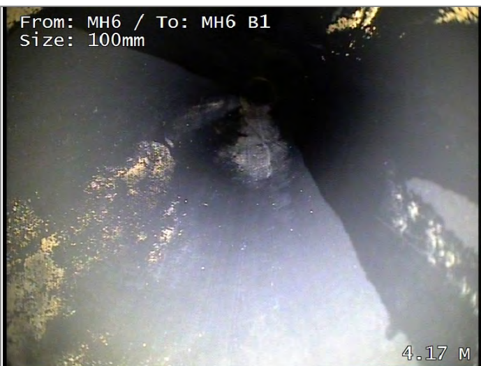
Finish node type, major connection without manhole, reference MH6 B1 REST BEND FOR SOIL STACK PIPE.
