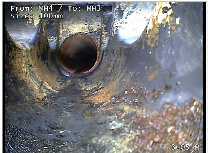
Finish node type, inspection chamber, reference MH3
