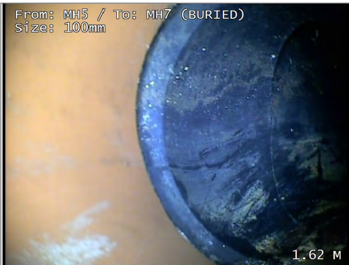
Line of drain/sewer deviates right
