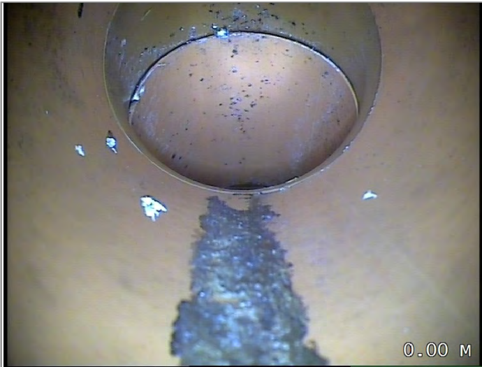
Start node type, inspection chamber, reference MH3
