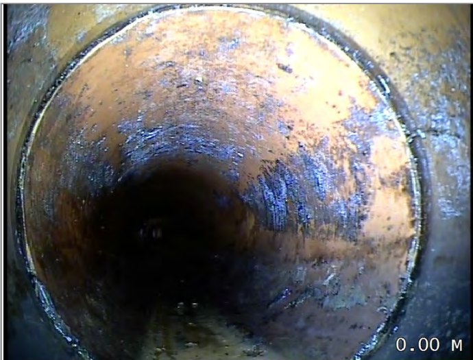
Start node type, inspection chamber, reference MH1
