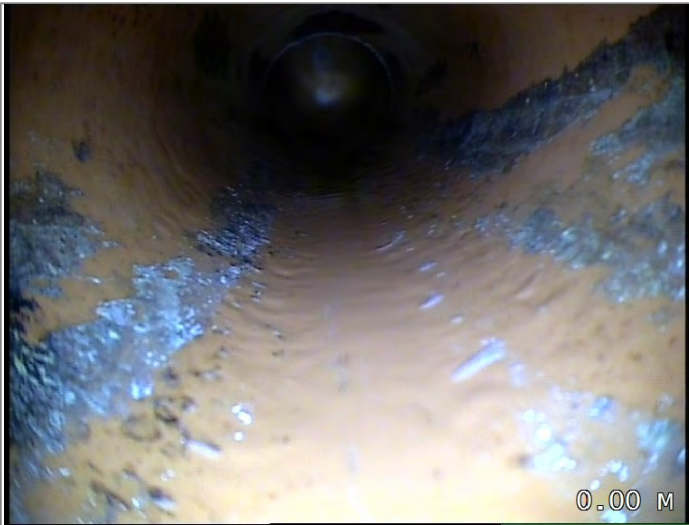
Start node type, inspection chamber, reference MH3
