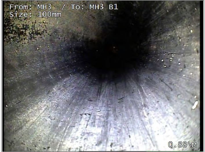
Finish node type, major connection without manhole, reference MH3 B1 REST BEND
