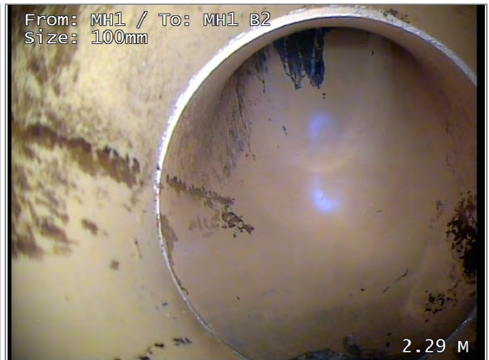
Line of drain/sewer deviates up
