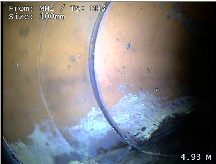
Line of drain/sewer deviates right
