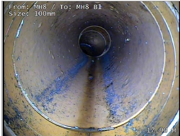
Line of drain/sewer deviates up
