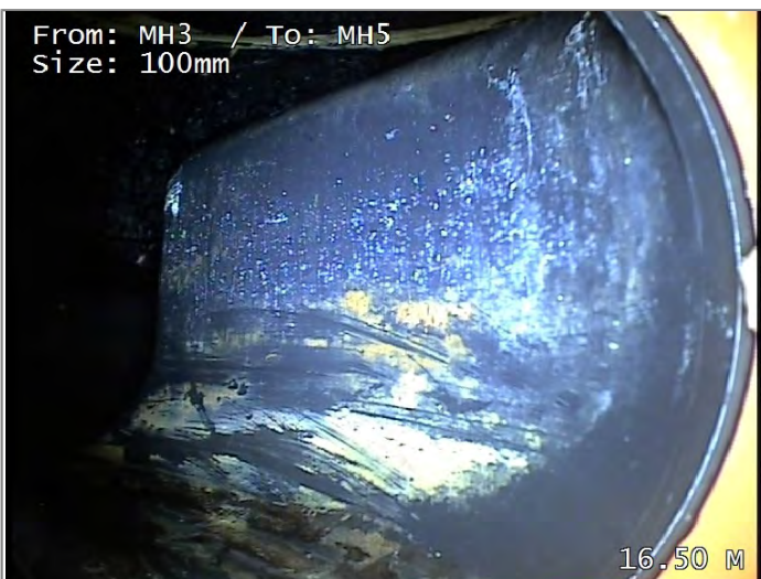
Finish node type, inspection chamber, reference MH5
