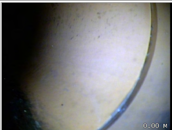
Start node type, inspection chamber, reference MH2
