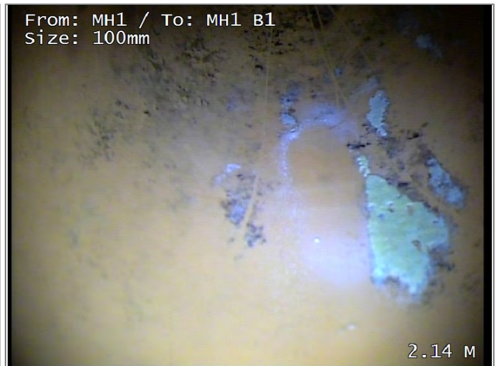
Line of drain/sewer deviates up
