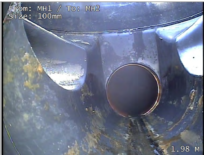
Finish node type, inspection chamber, reference MH2
