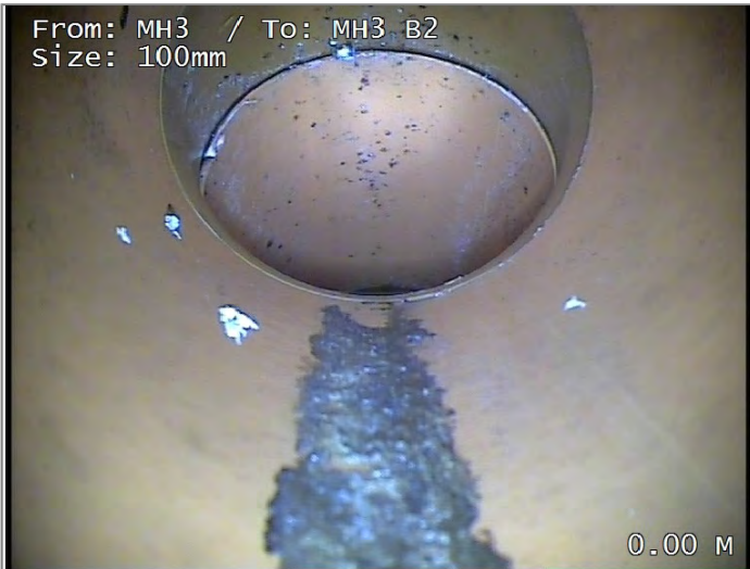
Line of drain/sewer deviates up
