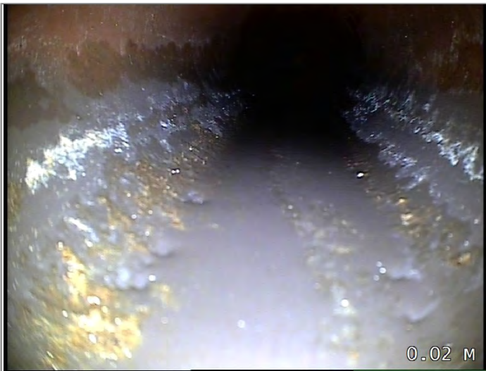
Start node type, inspection chamber, reference MH4
