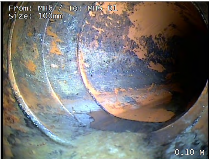
Line of drain/sewer deviates right
