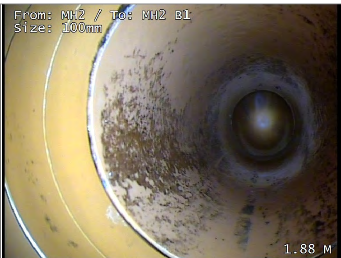
Line of drain/sewer deviates right
