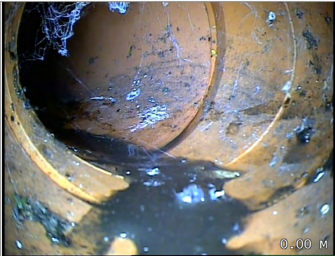
Start node type, inspection chamber, reference MH8
