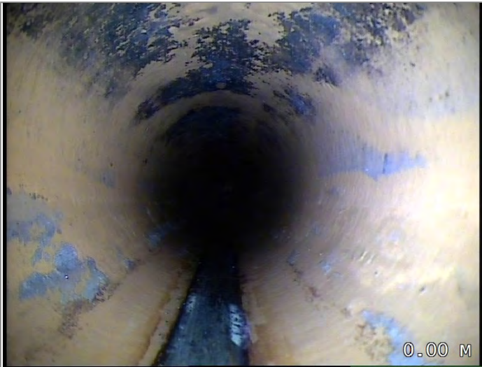
Start node type, inspection chamber, reference MH2
