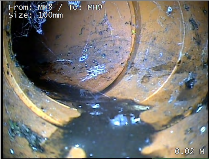
Line of drain/sewer deviates left
