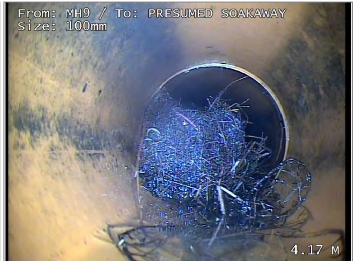
Roots mass 5% cross-sectional area loss
