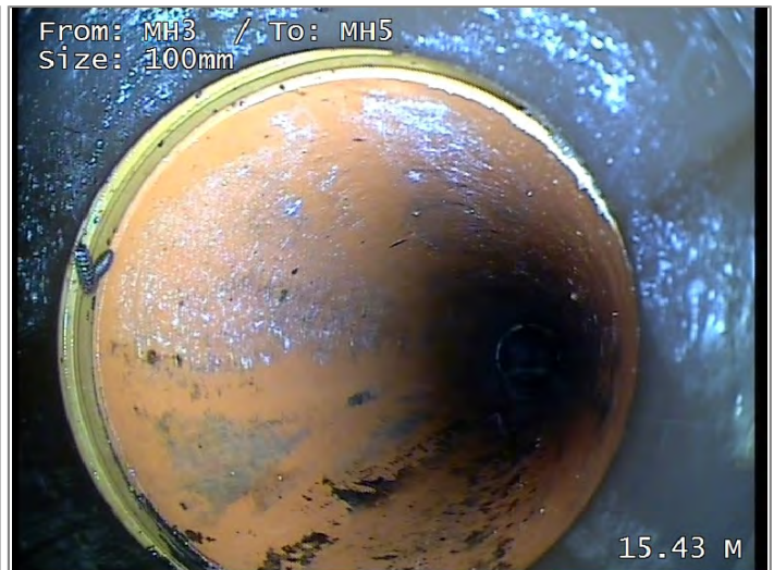
Line of drain/sewer deviates right
