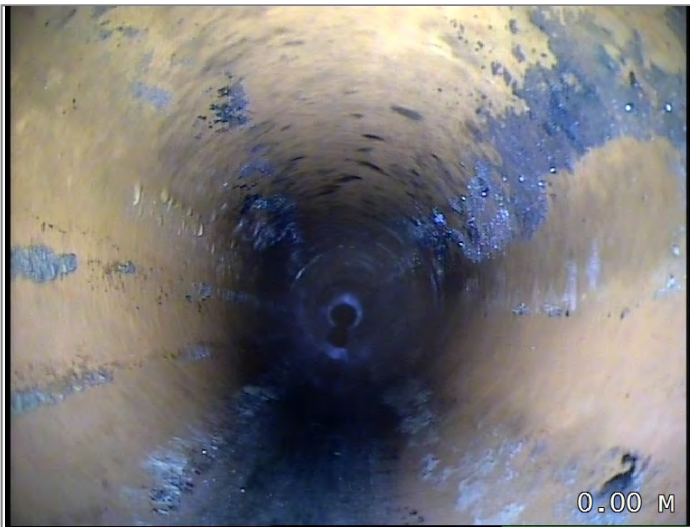
Start node type, inspection chamber, reference MH1
