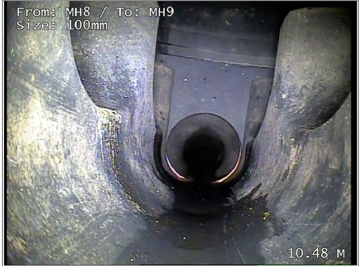
Finish node type, inspection chamber, reference MH9
