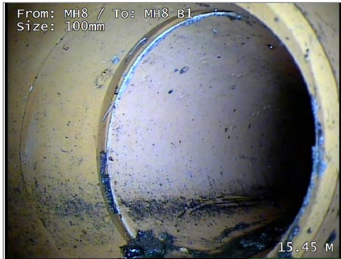
Line of drain/sewer deviates right
