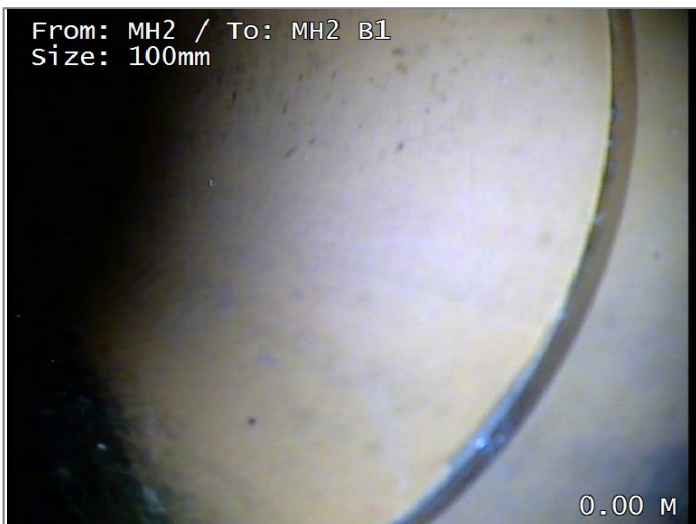
Line of drain/sewer deviates left
