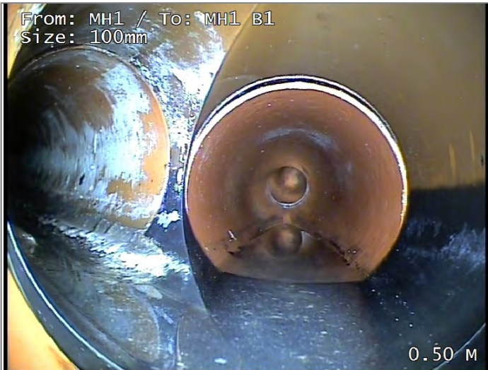
Junction at 9 o'clock, diameter 100mm - Remark: JUNCTION SERVES GULLY AT FRONT OF HOUSE.
