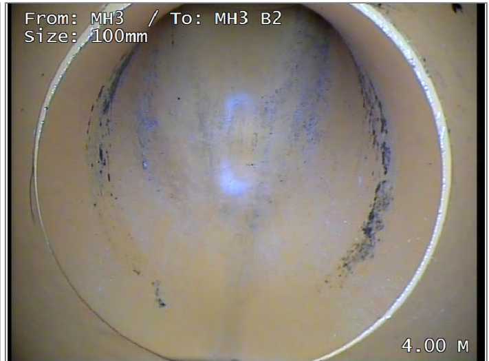
Line of drain/sewer deviates up
