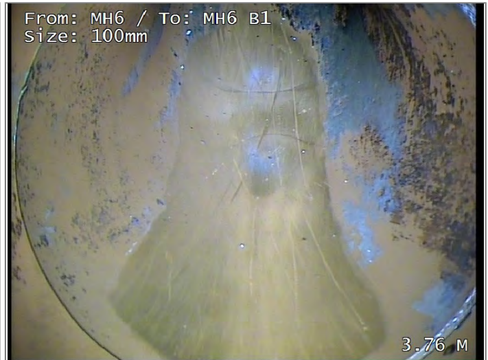
Line of drain/sewer deviates up
