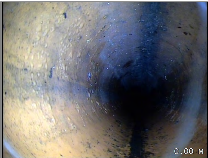
Start node type, inspection chamber, reference MH9
