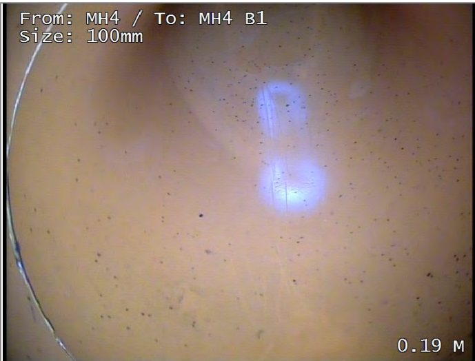
Line of drain/sewer deviates up
