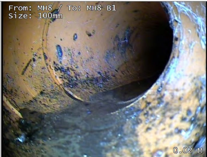
Line of drain/sewer deviates left
