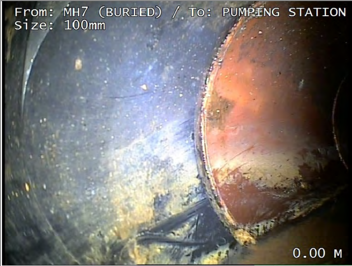
Line of drain/sewer deviates right
