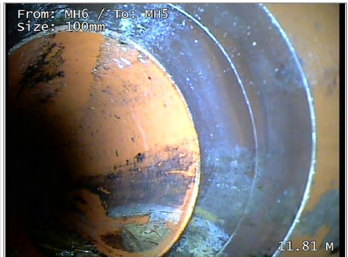
Line of drain/sewer deviates left
