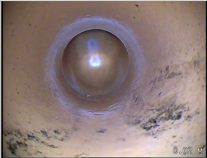
Start node type, inspection chamber, reference MH4
