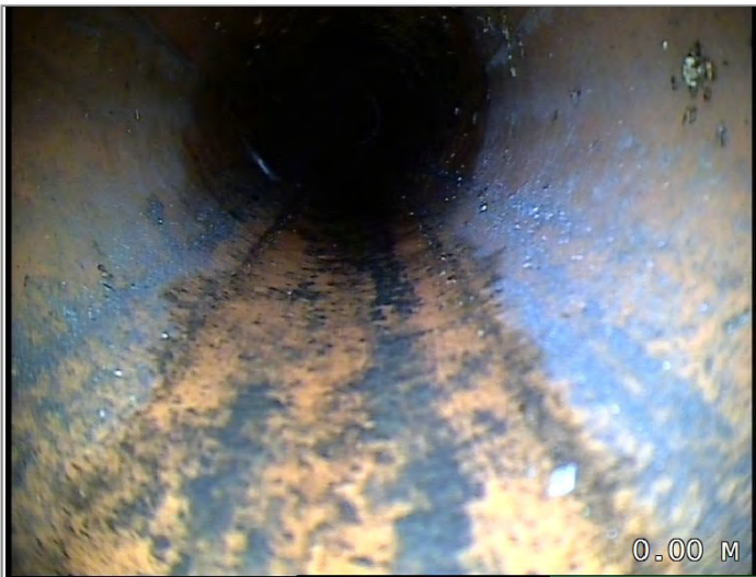
Start node type, inspection chamber, reference MH9
