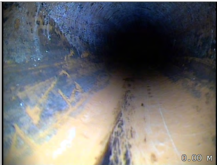
Start node type, inspection chamber, reference MH3
