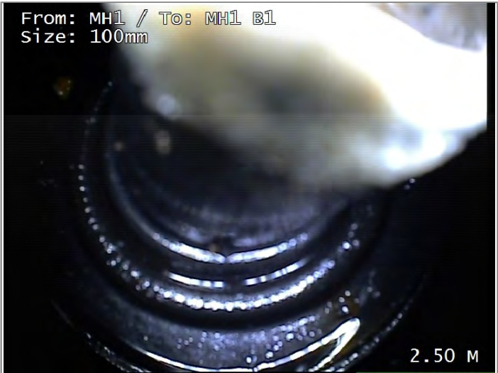
Finish node type, major connection without manhole, reference MH1 B1 REST BEND
