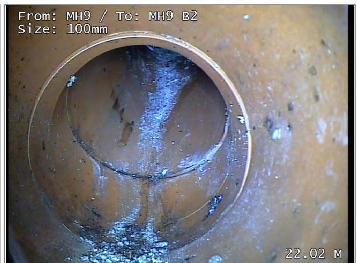
Line of drain/sewer deviates up
