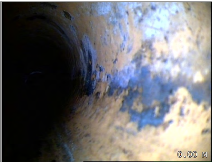
Start node type, inspection chamber, reference MH1
