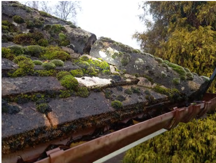
Plate 7 - Gap in ridge tile
