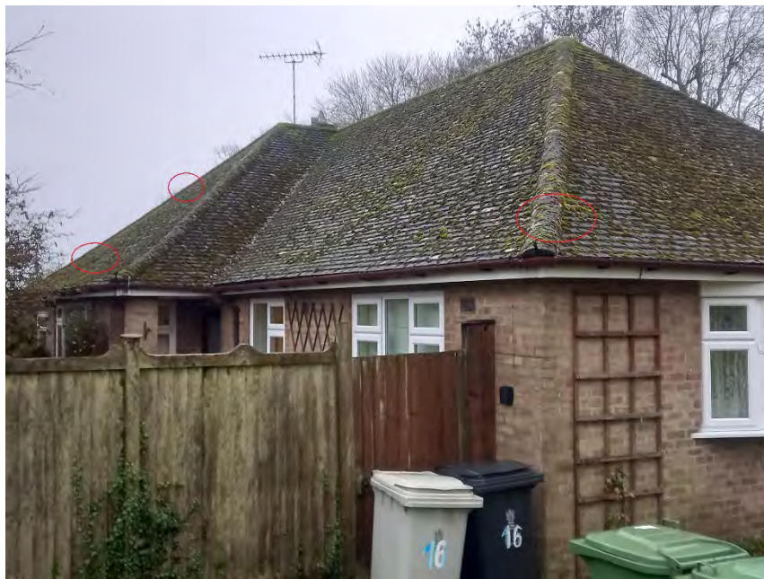
Plate 8 - Lifted ridge tiles at SE and gap in ridge tile at NE
