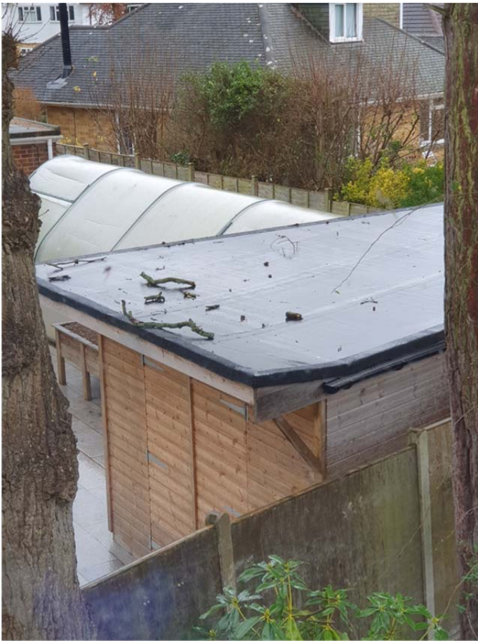
1 Debris that is regularly falling from Oak at present
