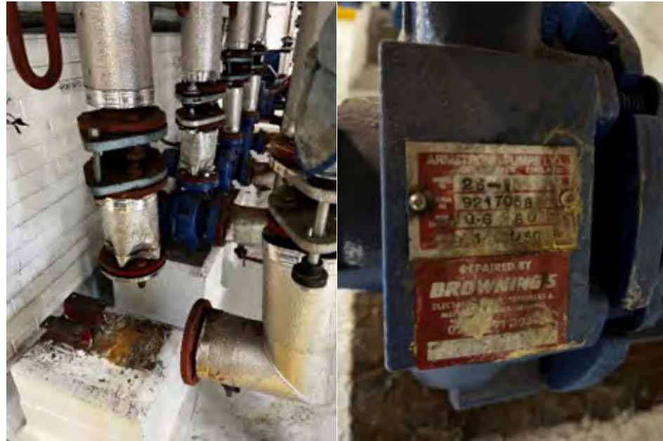
Existing secondary LTHW pumps (left), showing nameplate of one of the existing pumps (right)
