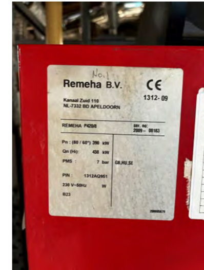
Existing boiler indicating year of manufacture 2009
