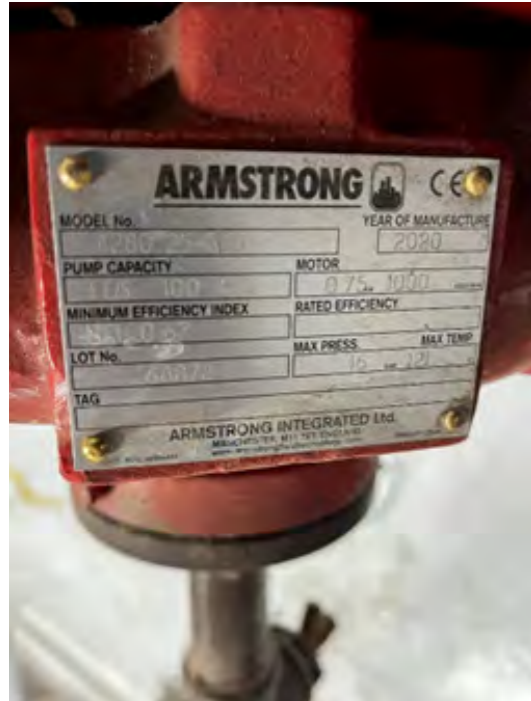
Image of a more recent replacement pump installed in 2020
