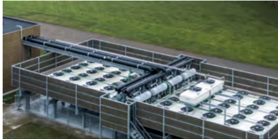
Large scale air source heat pump installation, Denmark. Image courtesy of Solid Energy.
