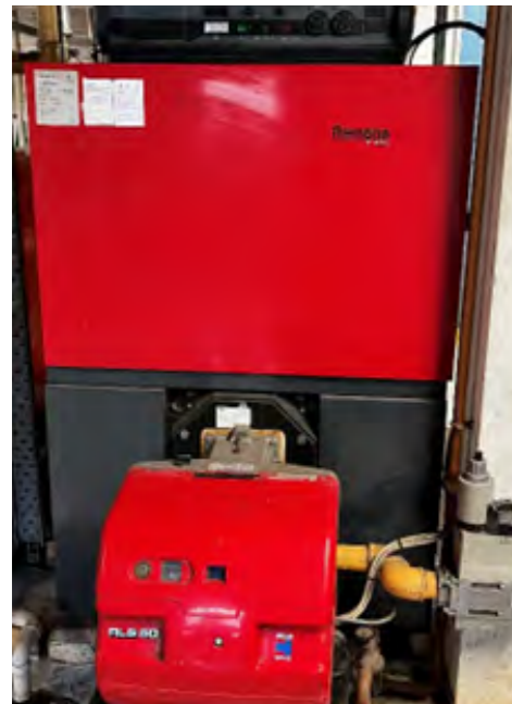
Existing Bexleyheath LTHW dual fuel boiler
