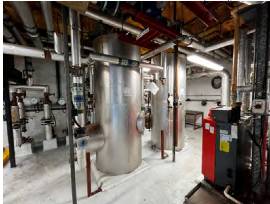
Domestic hot water calorifiers
