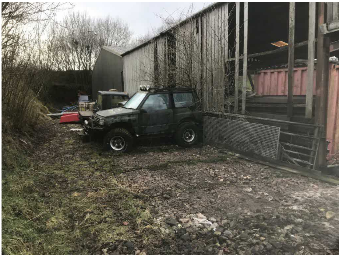
Note poor condition of cladding and steel frame.
