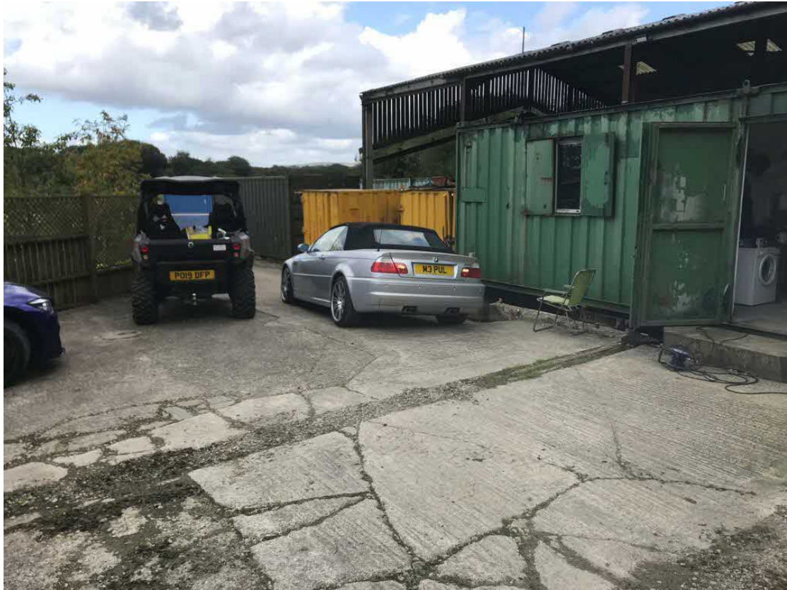
Note lack of gutters and downpipes and general poor condition of steel frame and cladding.
