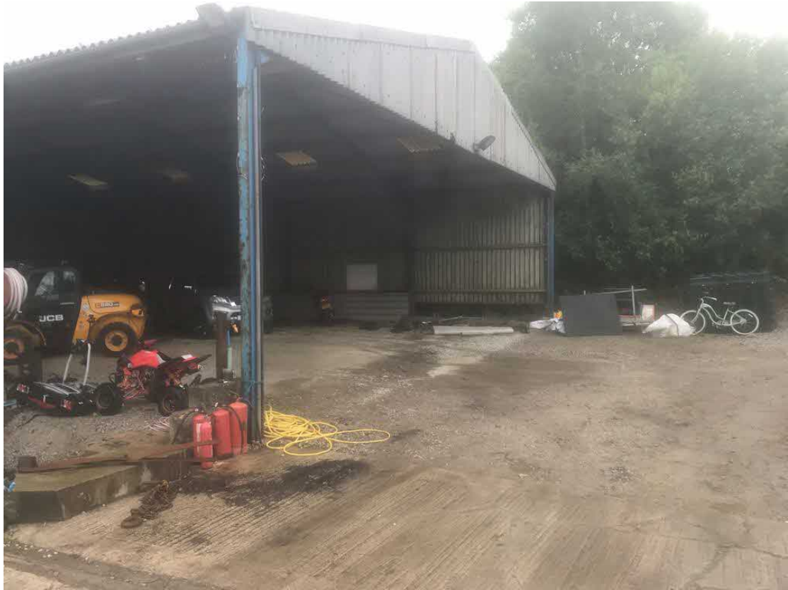
Note slender columns, lack of bracing and haunches and corrosion of steel frame.
