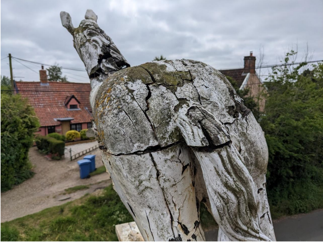
Photo 3 Horse at time of removal – it is at an angle following a storm
