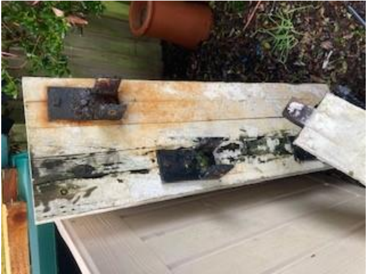
Photo 7 Plinth which has been retained and is yet to be repaired with stainless fittings proposed
