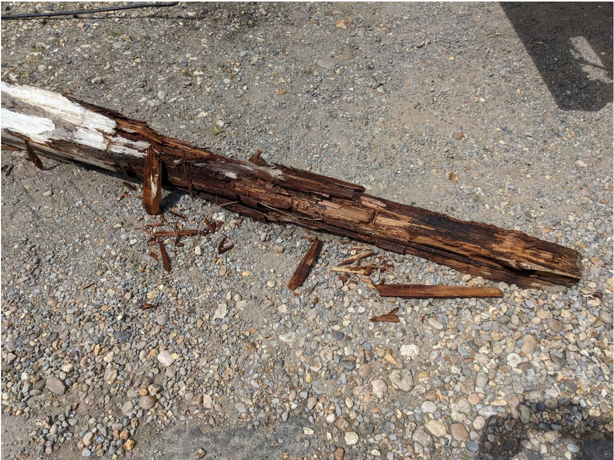
Photo 1 Base of the post showing rot – the post is to be replaced
