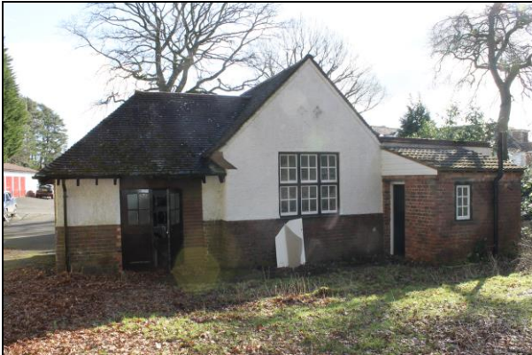
Plate 5:A: View of the rear (western) elevation of the structure, backing on to the semi-natural woodland
