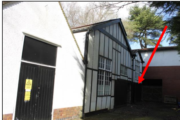
Plate 12:C: View of the front (eastern) elevation of the workshops with interior bat roost identified in 2020 and 2023
