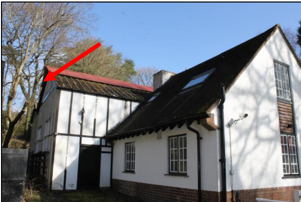
Plate 11: C: View of the rear of the offices and attached workshops. Long-eared bat roost access point indicated in 2020 and in use 2023
