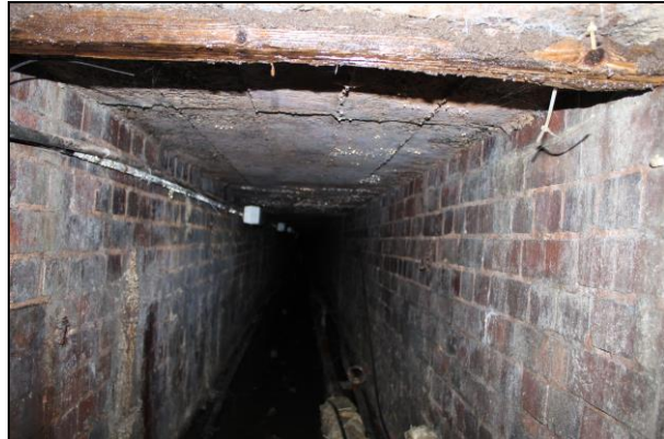
Plate 10:C: View of the service tunnel potentially suitable for a range of bat roosting use. Distant from the western (office cellar) end a confirmed summer use of these by lesser horseshoe bats has been observed in the summer of 2020 and again in 2023
