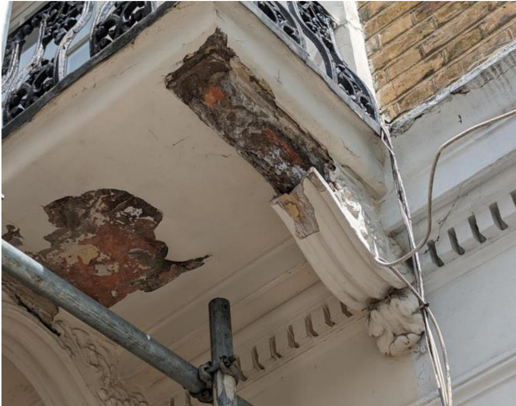
Figure 4.1: Existing state of disrepair to the balcony slab and bracket.
