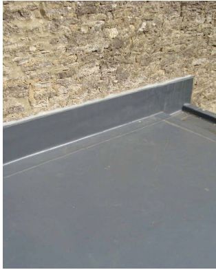
Single ply membrane roofing, in lead grey colour. Lead flashing to upstands, to LSA standard details.
