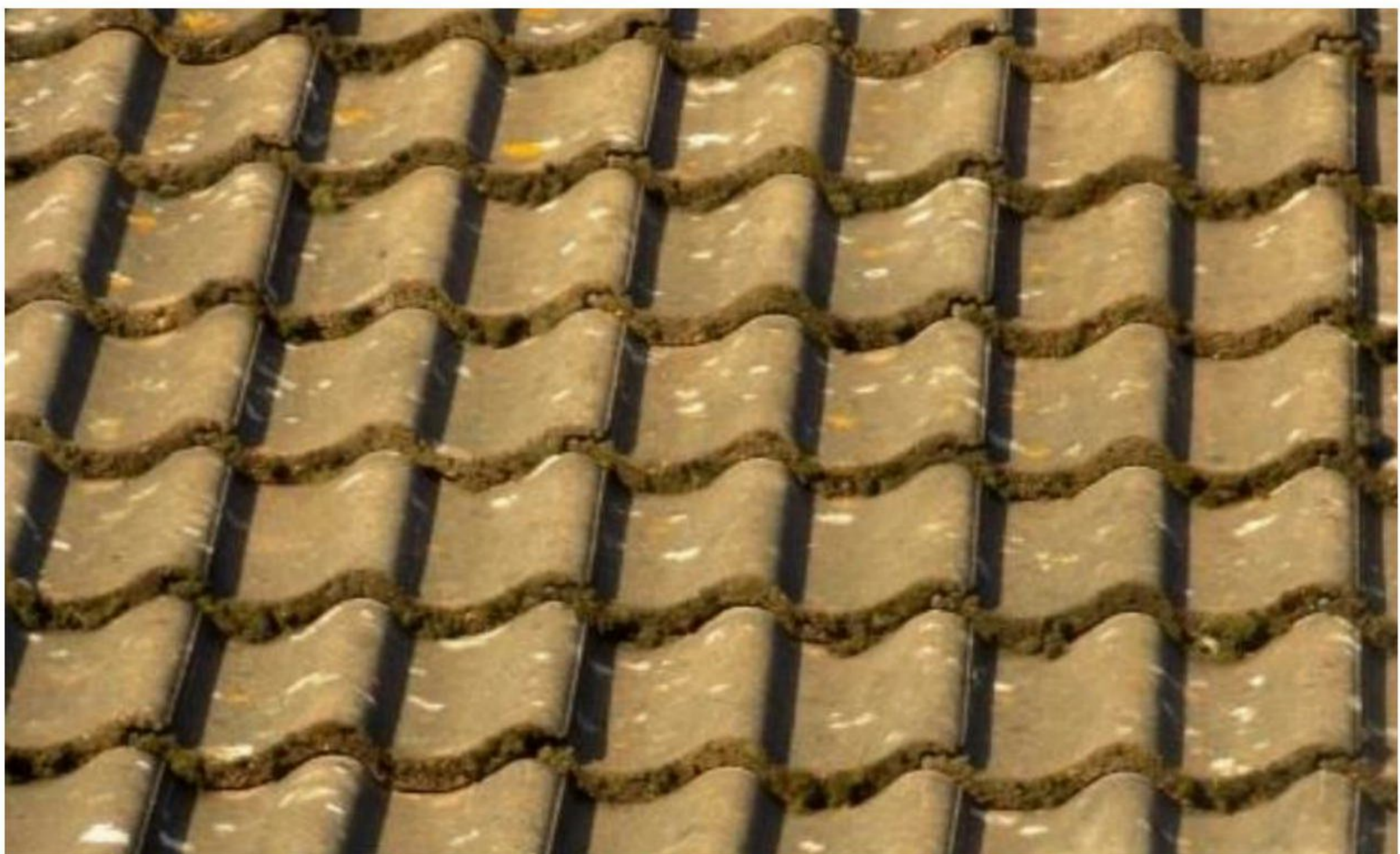
Image 4 – Close view of front roof coverings to demonstrate condition and lack of roosting features throughout
