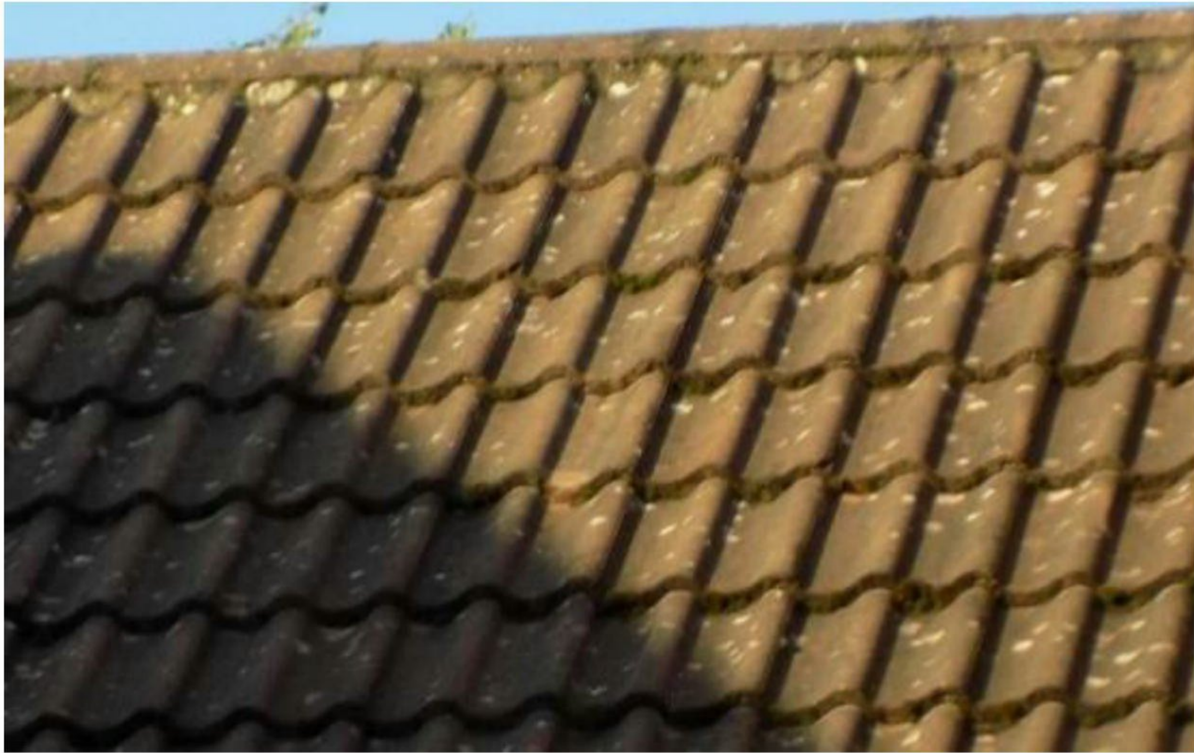
Image 5 – Close view of rear roof coverings to demonstrate condition and lack of roosting features throughout
