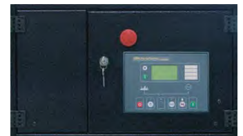
Deep Sea 7310 Control Panel
