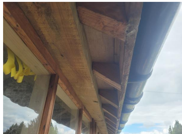
P6: Detail of the obstructed eaves
