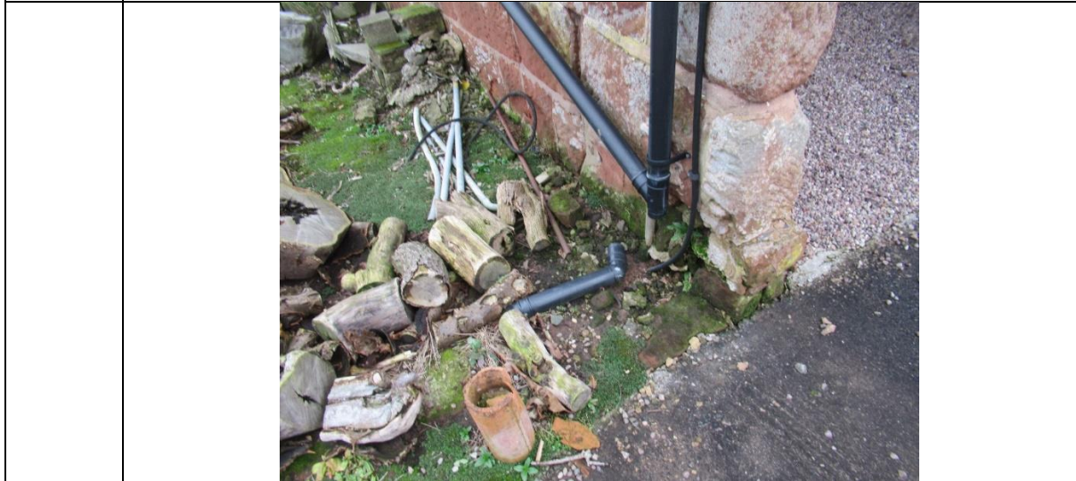
Disconnected shoe to drainpipe
