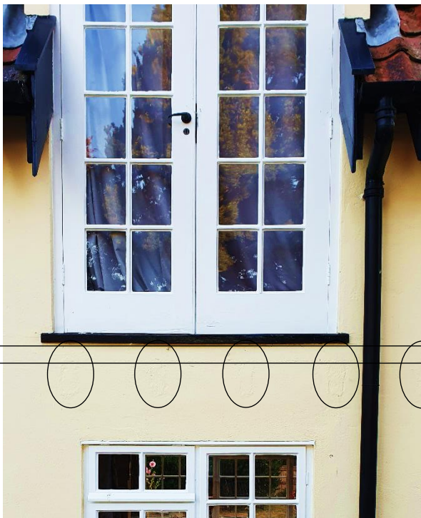
Figure 3 : photo of existing French doors at first floor showing ‘scars’ in the render of removed supports for a balcony structure. It is proposed to reinstate the balcony to make the existing French door arrangement safe for use by the occupants. See also Figure 4 which demonstrates the balcony originally extended wider than the French doors. The assumed dimensions of the original balcony are 3.6m wide x min. 750mm deep (to accommodate opening of doors).
