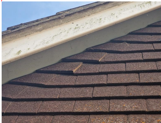
(Photo 1: Shows some of the potential roosting and access opportunities on the North elevation including elevated tiles and other appropriate gaps)
