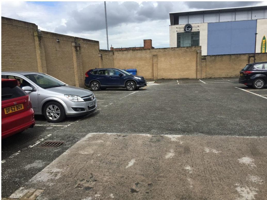
Fig 7. View north (note: gully adjacent parking space no.19)
