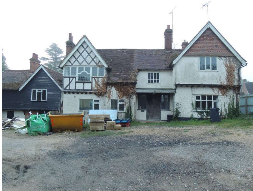
Photo 1: North-western elevation. The proposal is to refurbish the building to create two residential dwellings
