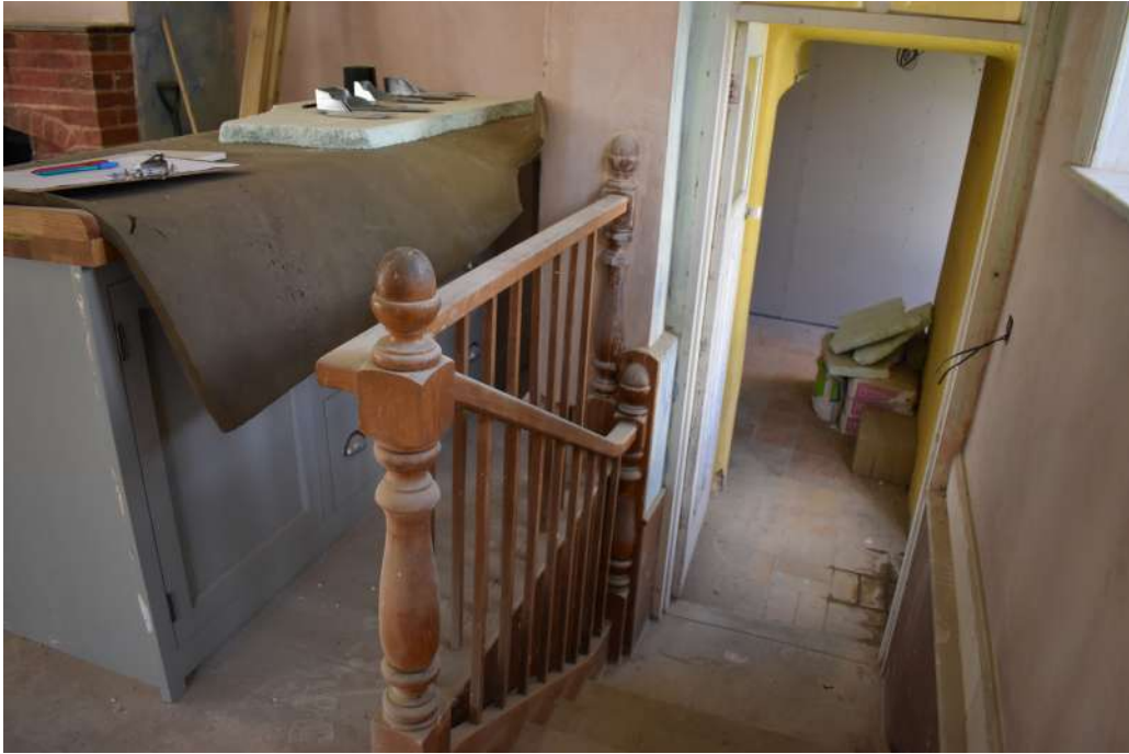
Photograph 34 Detail of staircase with bannister and newel posts in room 12. Photograph taken facing north-west.
