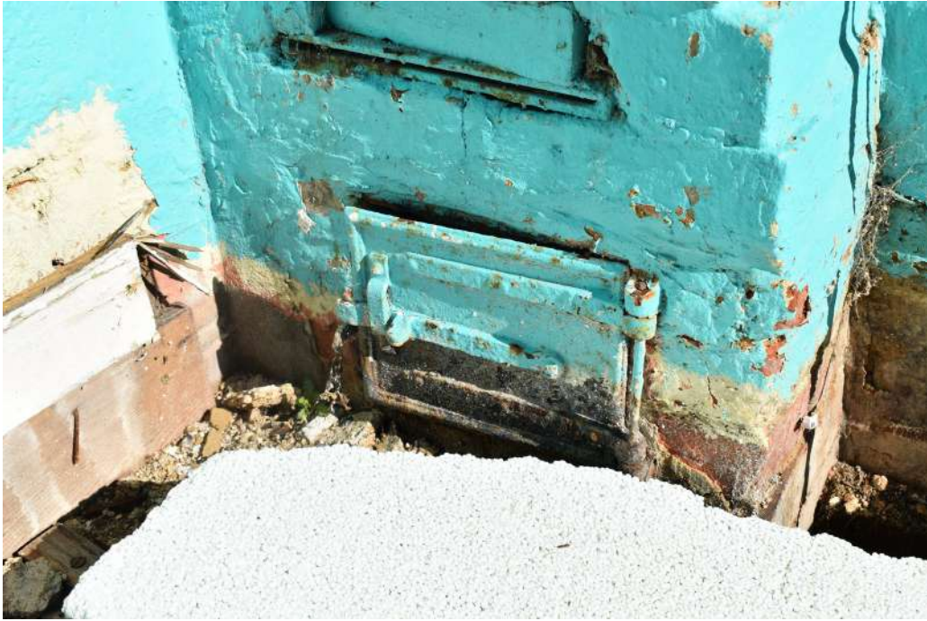
Photograph 15 Detail of clean out door in south-west elevation. Photograph taken facing north.
