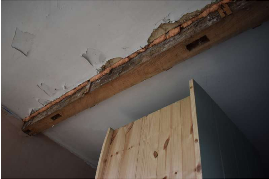
Photograph 32 Detail of empty mortices in girding-beam above window in room 11. Photograph taken facing south-west.
