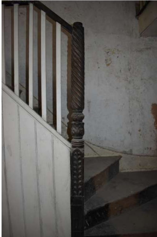
Photograph 30 Detail of newel post on staircase in room 10. Photograph taken facing south-east.
