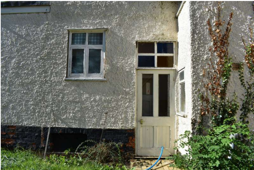
Photograph 11 Detail of blocked opening, window and door on north-east elevation. Photograph taken facing south-west.
