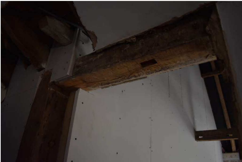
Photograph 49 Detail of empty mortice in wall-plate in room 21. Photograph taken facing south-west.
