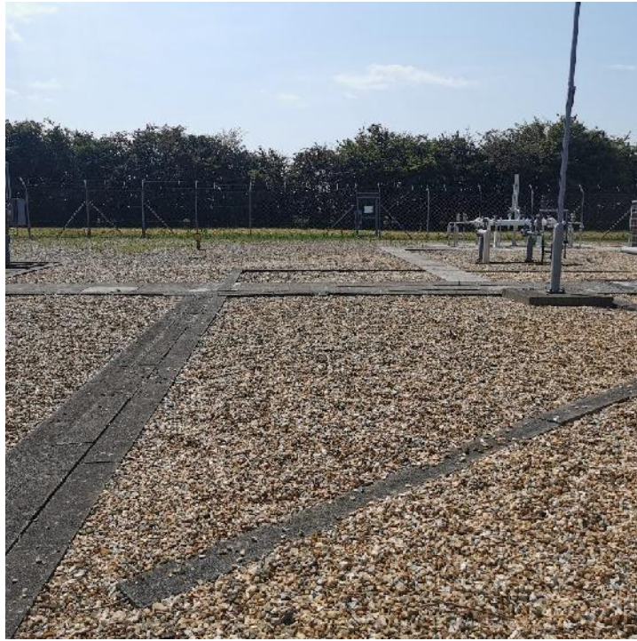
Photograph 13 – Gravel hardstanding with cable troughing
