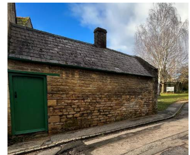
Fig 19. External door to kitchen to be infilled internally & chimney stack to be removed
