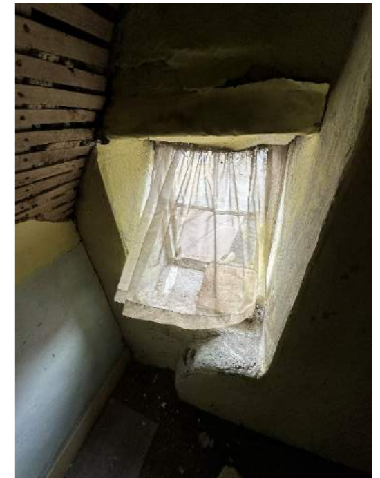
Fig 27. Existing attic room window condition
