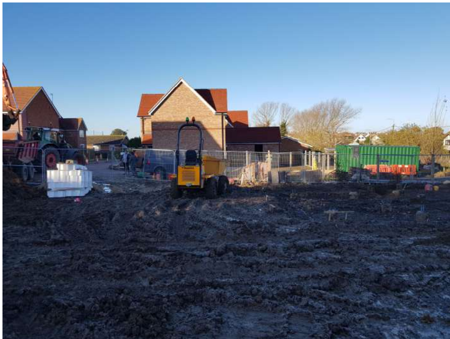
Looking west/northwest across the central area of the northeast area of the site that is proposed for plots 5 to 8. The unfinished plot 3 is in the background.
