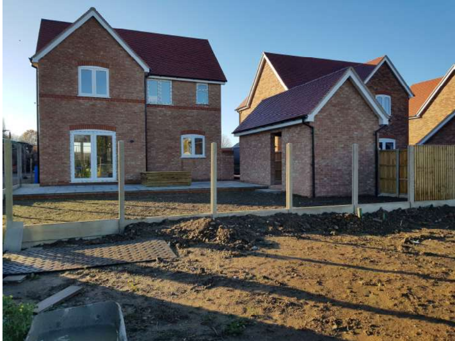
Looking southwest from the northeast area of the site at the incomplete plot 3. The adjacent occupied plot 2 is in the background.
