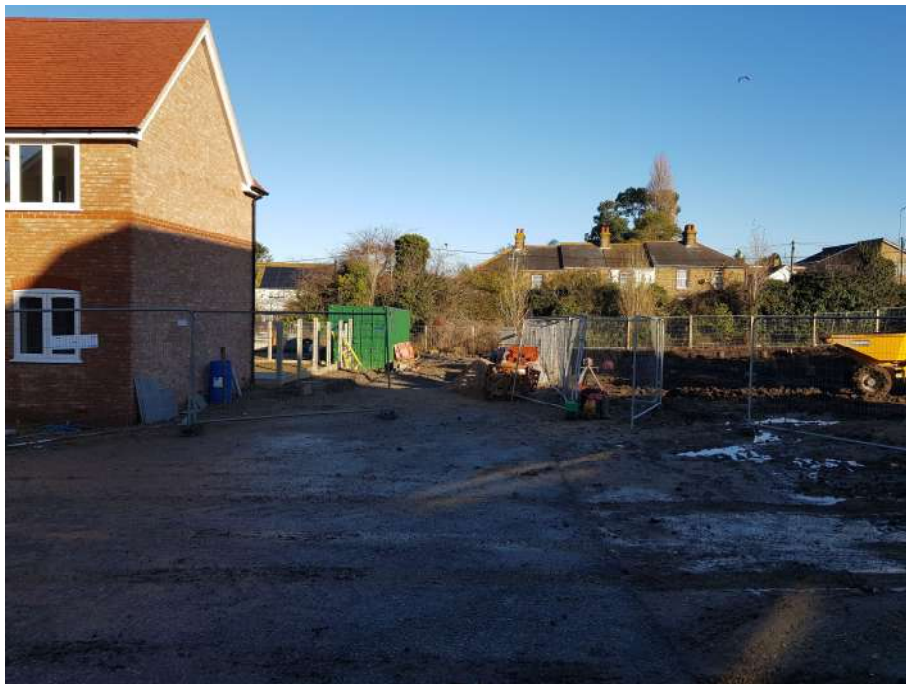
Looking north/northeast from the centre of the site at the location of the proposed access road to plot 4. The parking areas to plots 5 to 8 will be on the right and the unfinished plot 3 is on the left.
