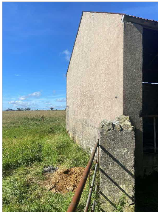
PHOTOGRAPH 2: View of the trial pit's location immediately adjacent to the southern-eastern gable end of the building
