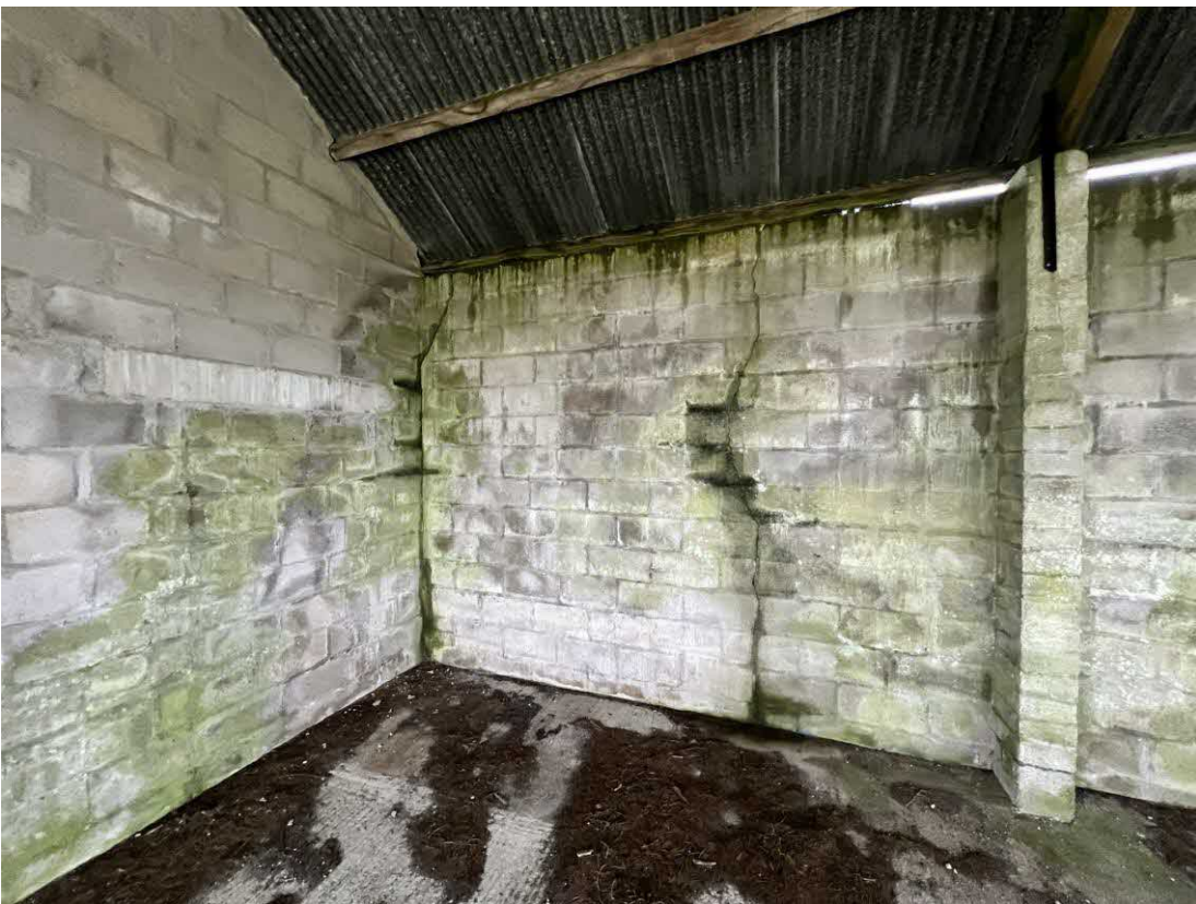
Figure 4 – Vertical cracking to south elevation due to thermal movement.
