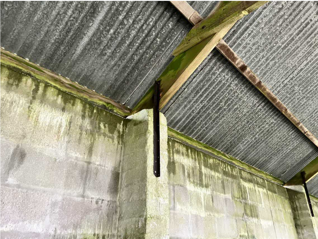
Figure 2 – Trusses supported by solid block piers also providing buttressing to south wall.
