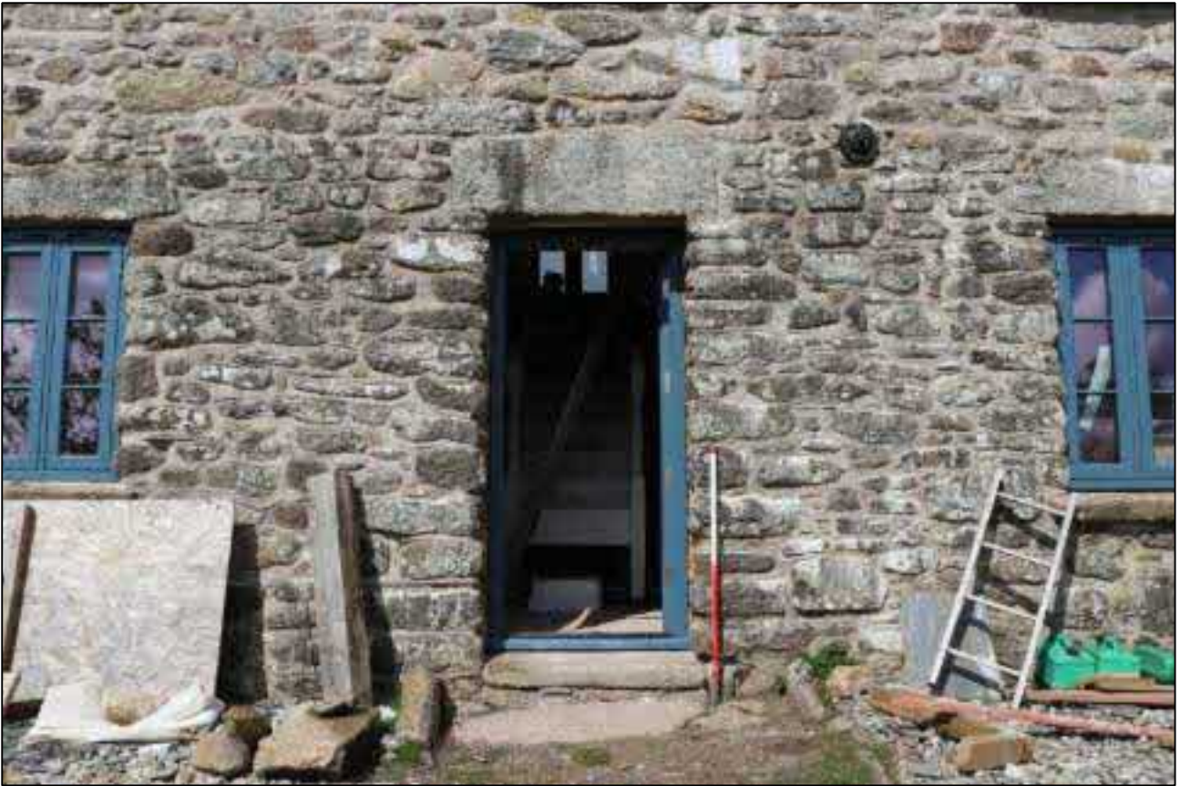
39. THE MAIN ACCESS TO CENTRAL BAY OF HOUSE; VIEWED FROM THE EAST (SCALE 1M).
