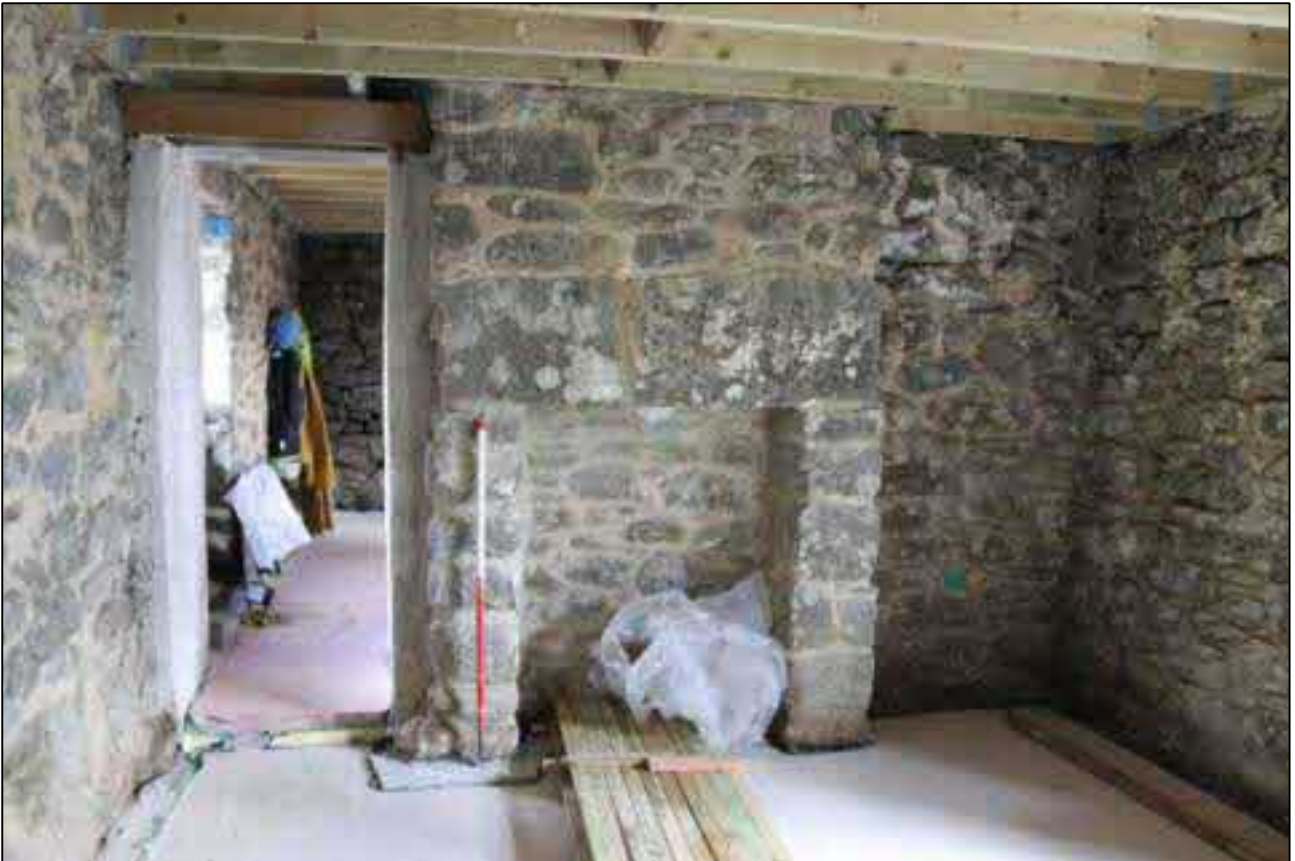
51. THE SHALLOW FIREPLACE AT THE NORTH END OF THE CENTRAL BAY; VIEWED FROM THE SOUTH (SCALE 1M).
