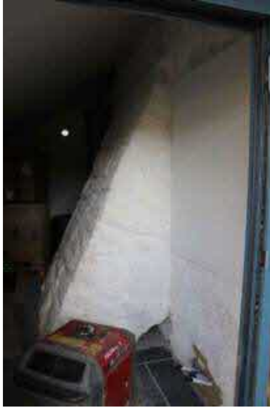
47. THE GRANITE BUTTRESS TO THE SOUTH END OF THE WEST ELEVATION, NOW WITH A MODERN PLANT ROOM; VIEWED FROM THE SOUTH.
