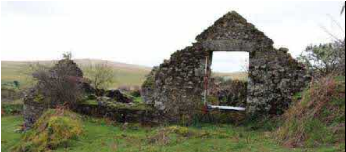
FIGURE 19: THE NORTH-EAST ELEVATION OF BARN, WITH A FIRST-FLOOR LOADING DOOR TO THE WEST END; VIEWED FROM THE NORTH-WEST (SCALE 2M).
