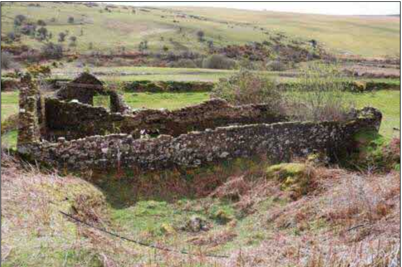
16. THE WEST EXTERNAL ELEVATION ABUTTED BY POSSIBLE HORSE WHIM; VIEWED FROM THE WEST (SCALE 1M).
