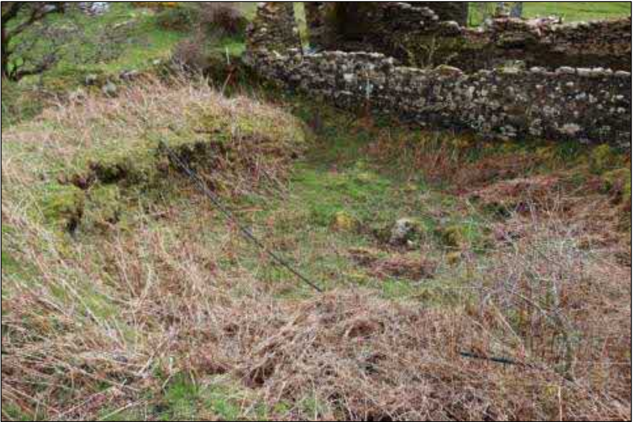
17. THE WEST EXTERNAL ELEVATION ABUTTED BY POSSIBLE HORSE WHIM; VIEWED FROM THE WEST (SCALE 1M).
