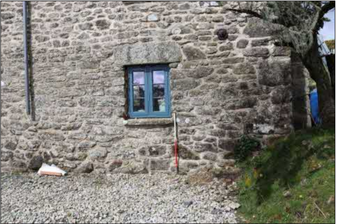
41. THE NORTH END OF EAST ELEVATION, THIS WINDOW OPENING IN A BLOCKED DOORWAY; VIEWED FROM THE EAST (SCALE 1M).
