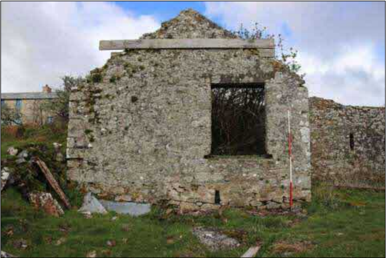
9. THE EAST FACING ELEVATION OF B1B WITH LARGE RECTANGULAR WINDOW; VIEWED FROM THE NORTH-EAST (SCALE 2M).
