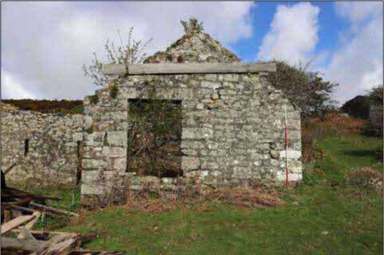
2. THE EAST ELEVATION OF B1C WITH LARGE SQUARE WINDOW; VIEWED FROM THE EAST (SCALE 2M).
