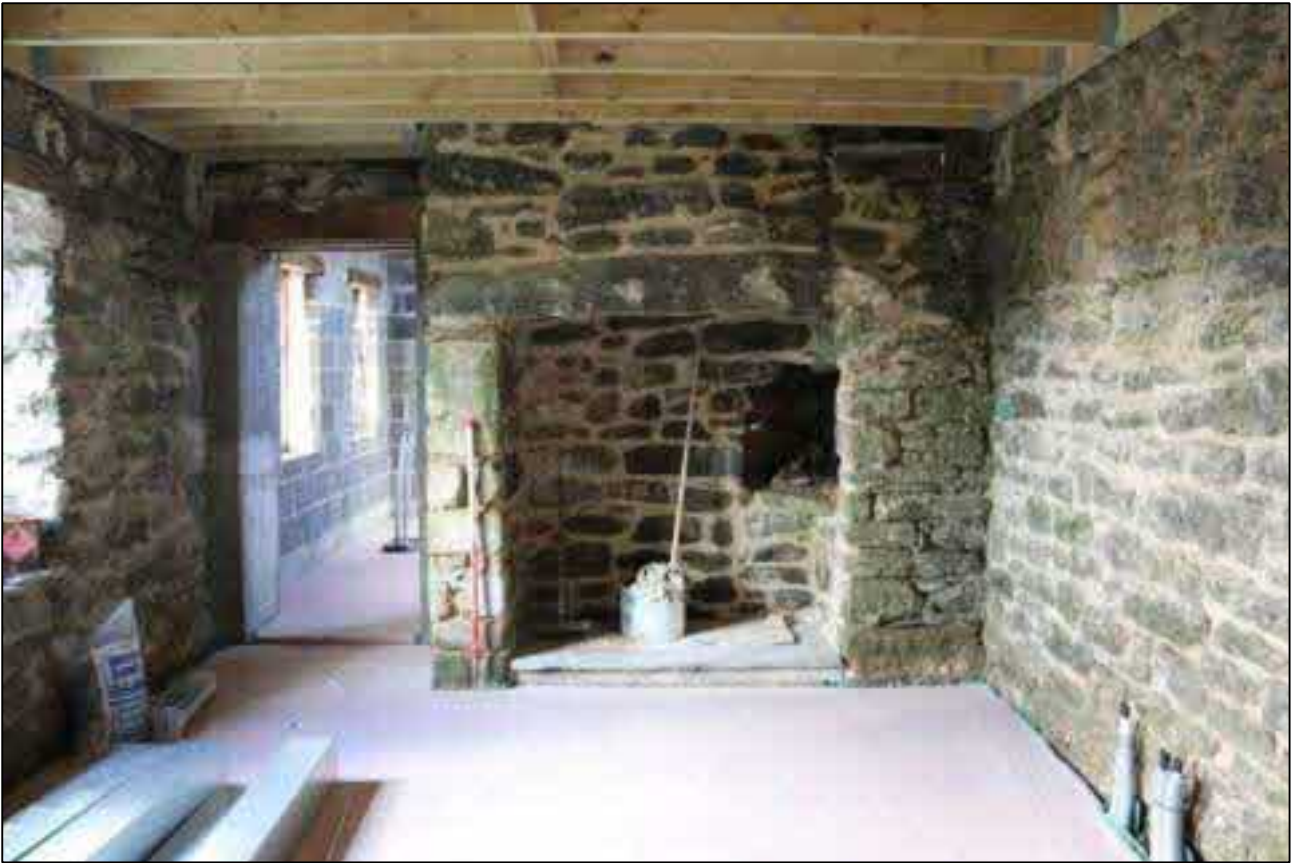
55. THE STACK TO SOUTH BAY WITH LARGE CLOAM OVEN TO RIGHT; VIEWED FROM THE NORTH (SCALE 1M).
