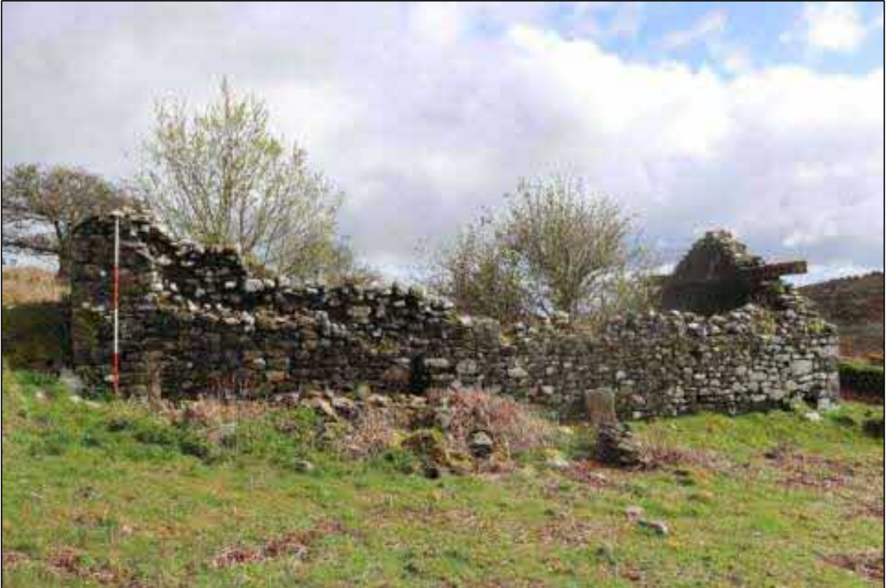
10. THE SOUTH-WEST ELEVATION SHOWING NO DISTINCT JOIN BETWEEN B1A AND B1B; VIEWED FROM THE SOUTH (SCALE 2M).
