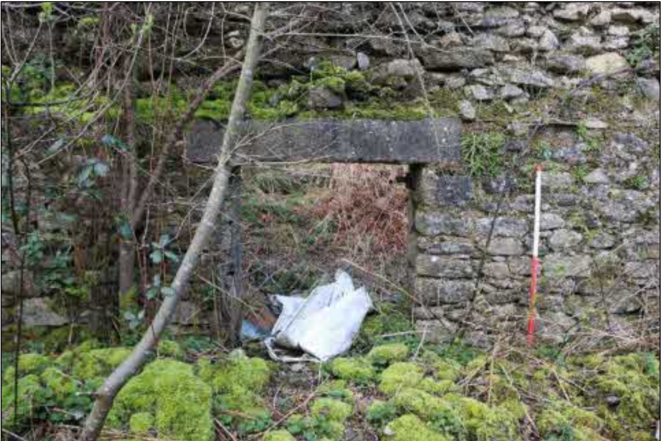
31. THE INTERNAL FACE OF ALTERED OPENING D6 TO WEST ELEVATION OF B1A; VIEWED FROM THE SOUTH-EAST (SCALE 1M).
