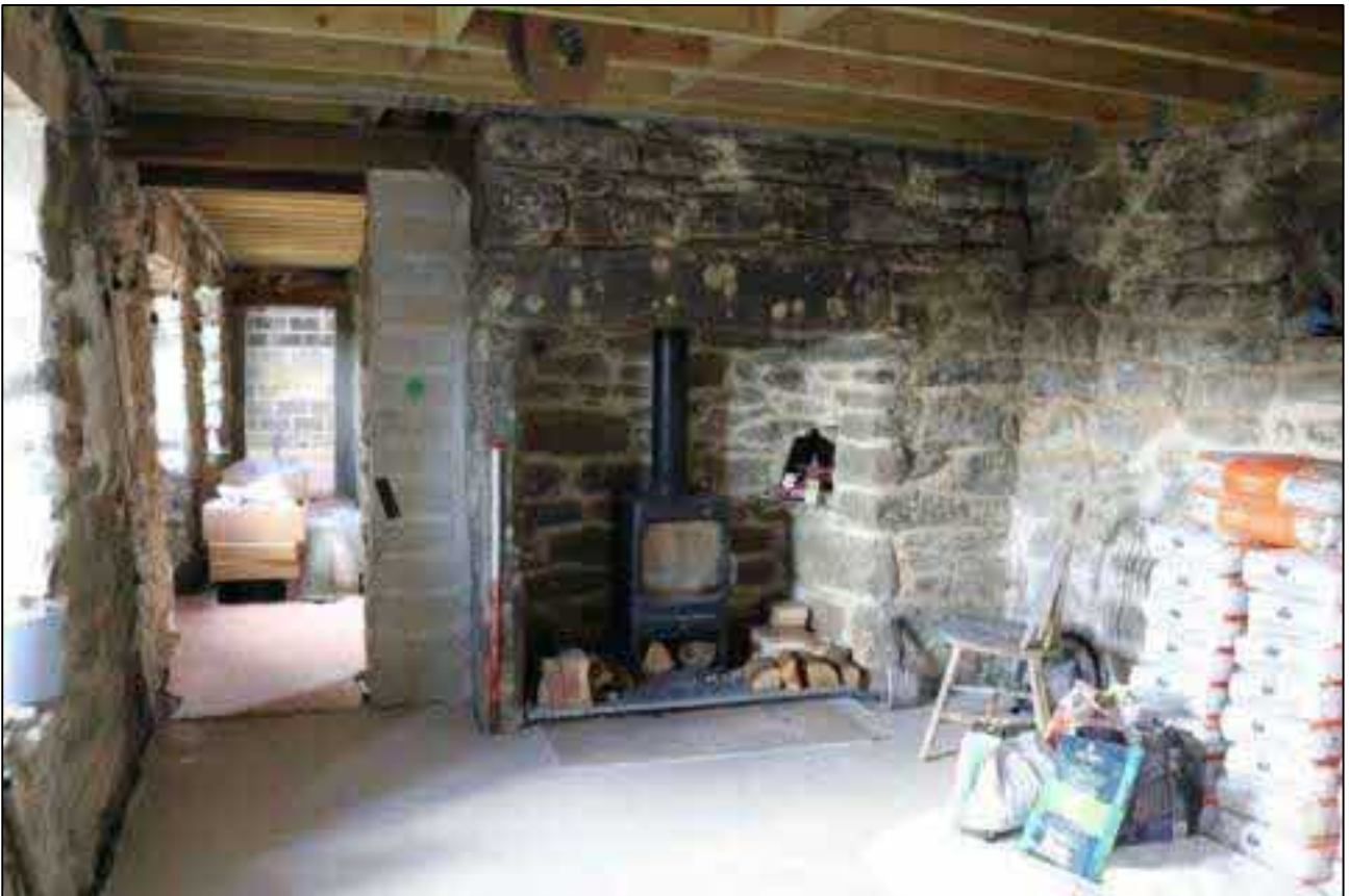
52. THE LARGE STACK TO THE SOUTH END OF THE CENTRAL BAY, CLOAM OVEN TO RIGHT; VIEWED FROM THE NORTH (SCALE 1M).
