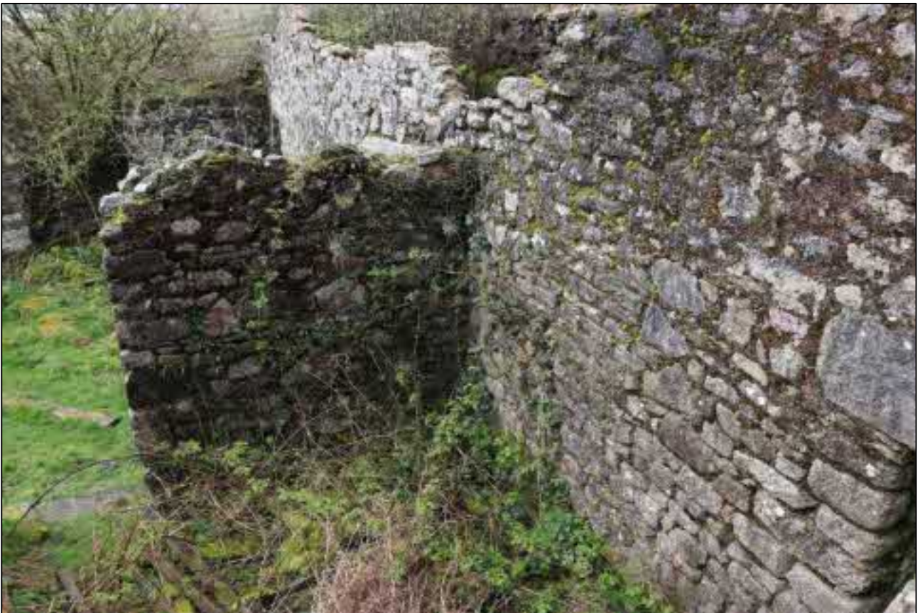
26. THE SOUTH INTERNAL ELEVATION OF B1C CLEARLY ABUTS B1A; VIEWED FROM THE NORTH.
