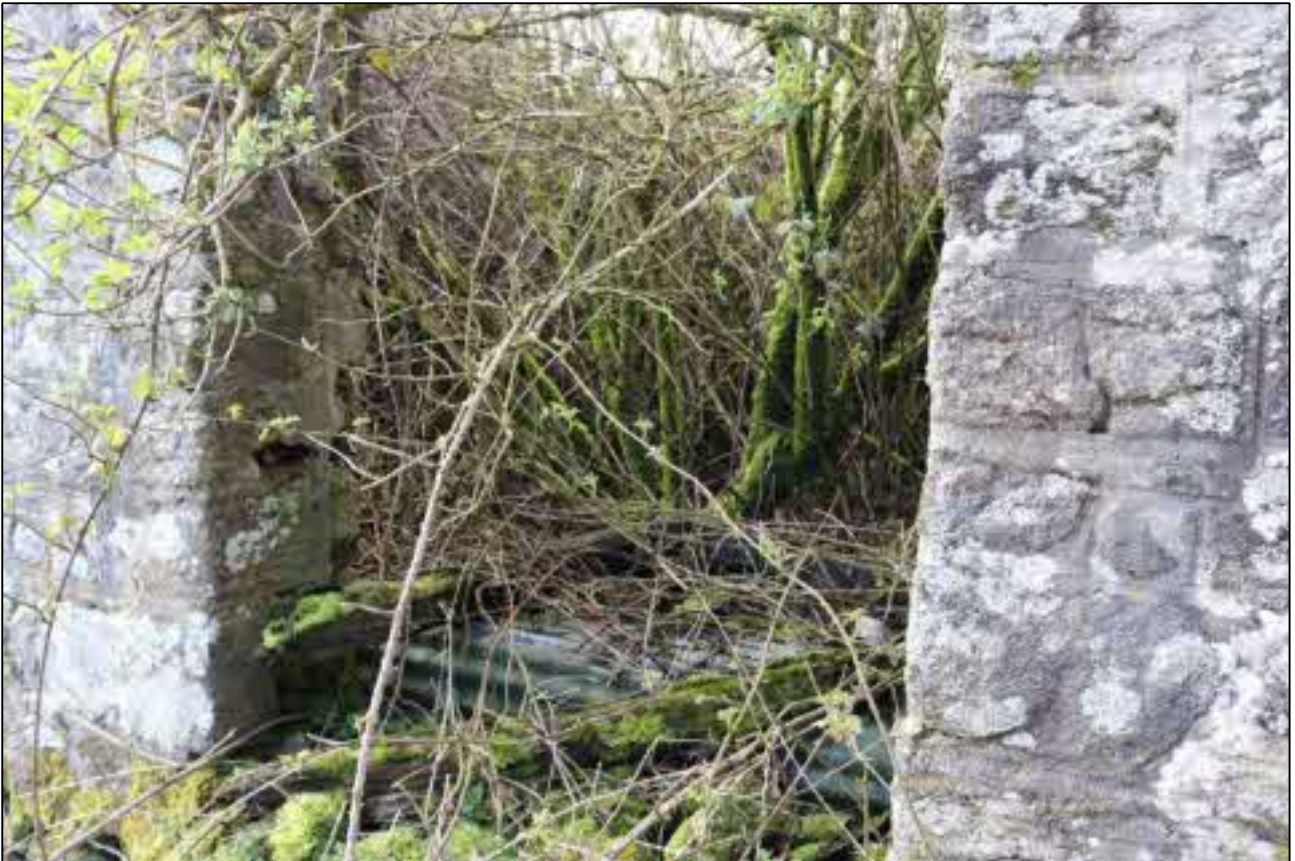
35. D4 OPENING TO B1B, THE DOORFRAME FALLEN OVER BUT IN SITU; VIEWED FROM THE NORTH-WEST.
