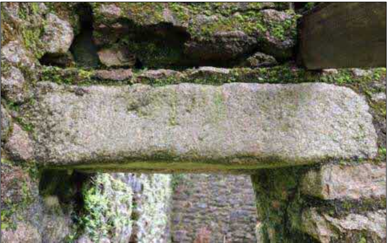
34. THE GRANITE LINTEL TO D1, LEADING FROM B1A TO B1C; VIEWED FROM THE WEST.
