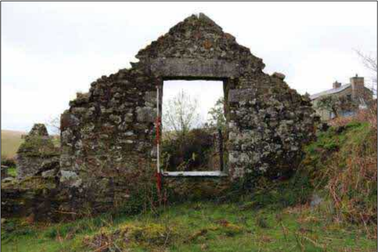
19. THE FIRST-FLOOR LOADING DOOR IN THE NORTH GABLE OF B1A; VIEWED FROM THE NORTH (SCALE 2M).
