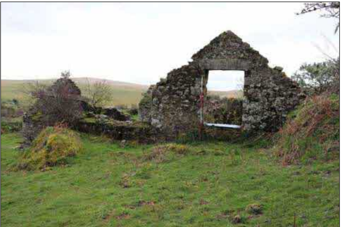
20. THE NORTH-EAST ELEVATION OF THE BARN; VIEWED FROM THE NORTH-WEST (SCALE 2M).
