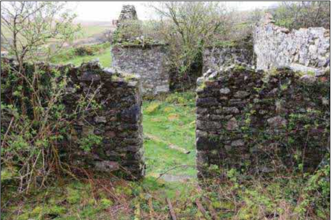
23. D5 IN B1C, LOOKING THROUGH TO D4 IN B1B; VIEWED FROM THE NORTH.
