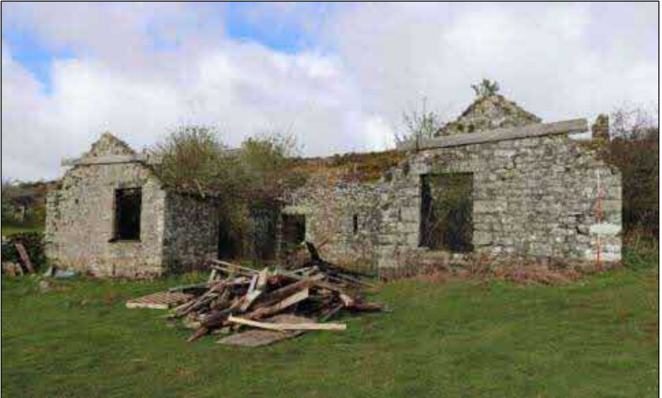
1. THE EAST ELEVATION OF THE BARN; VIEWED FROM THE NORTH-EAST (SCALE 2M).
