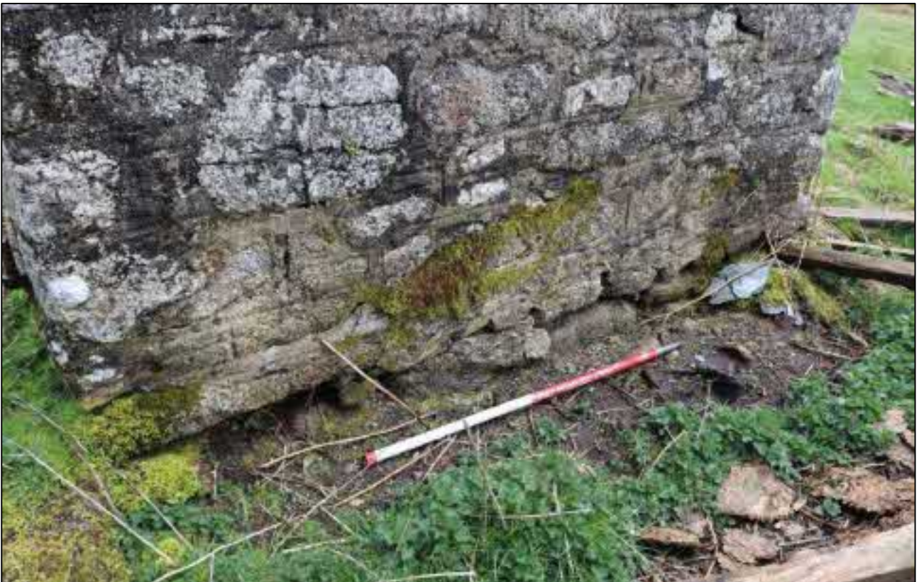
28. THE BASE OF WALL TO B1C LOOKING EXPOSED AND RAGGED, GROUND LEVELS ALTERED AS CONCRETE RIBBON POINTING DOES NOT CONTINUE; VIEWED FROM THE SOUTH-WEST (SCALE 1M).
