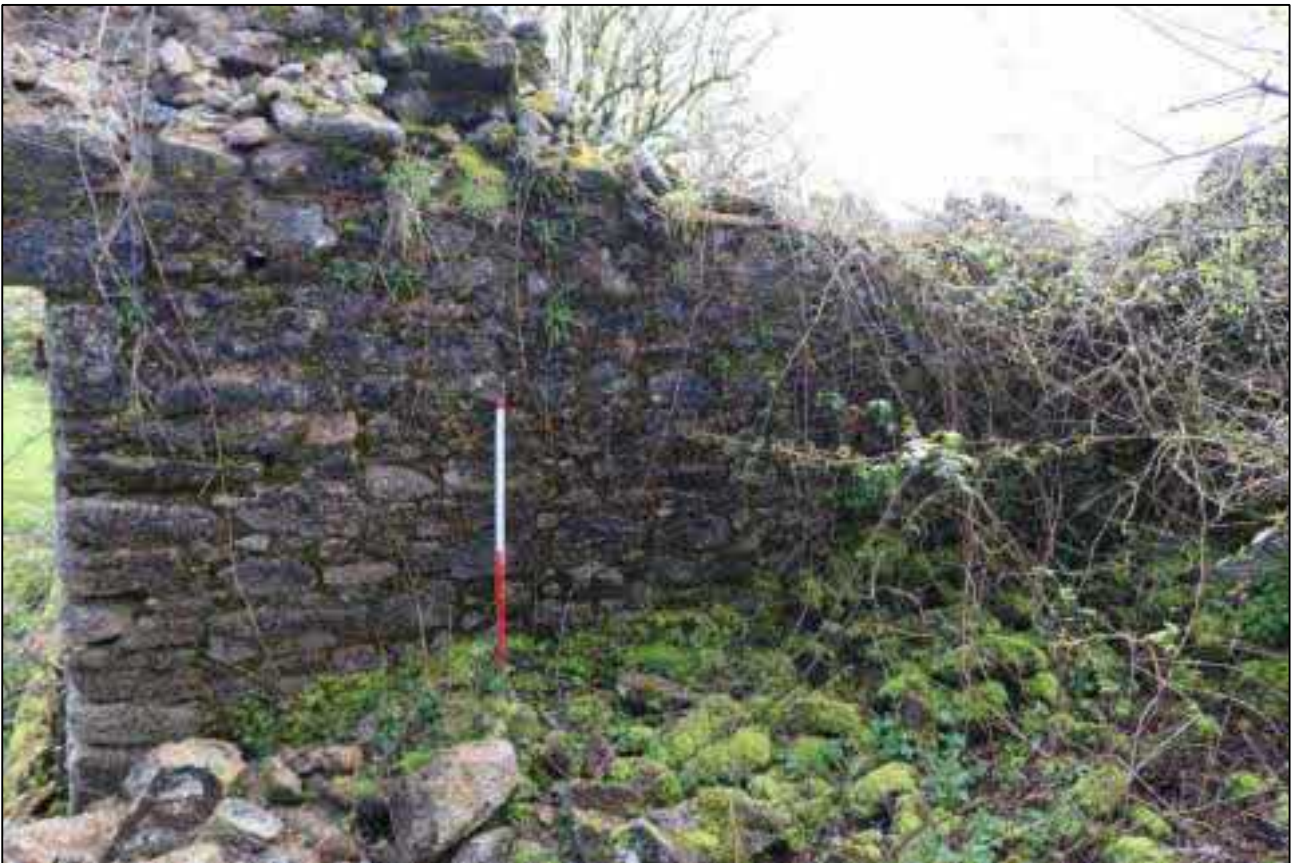
30. THE SOUTH-EAST CORNER OF B1A, NO EVIDENCE OF AN OPENING IT TO B1B; VIEWED FROM THE WEST (SCALE 1M).
