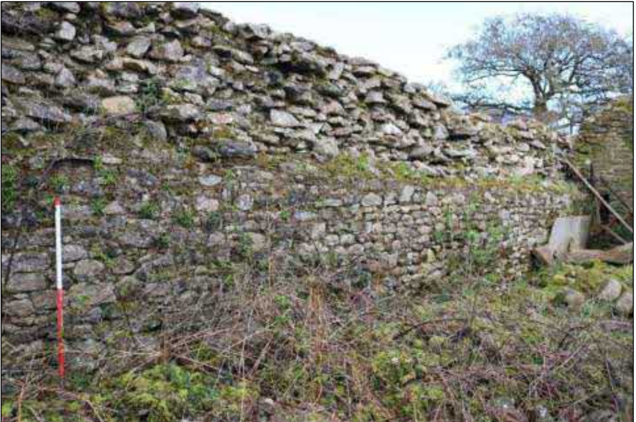
33. THE INTERNAL WEST ELEVATION SHOWING WHERE THE INNER FACE OF THE WALL ABOVE THE TIMBER LACING HAS COLLAPSED; VIEWED FROM THE SOUTH-EAST (SCALE 1M).
