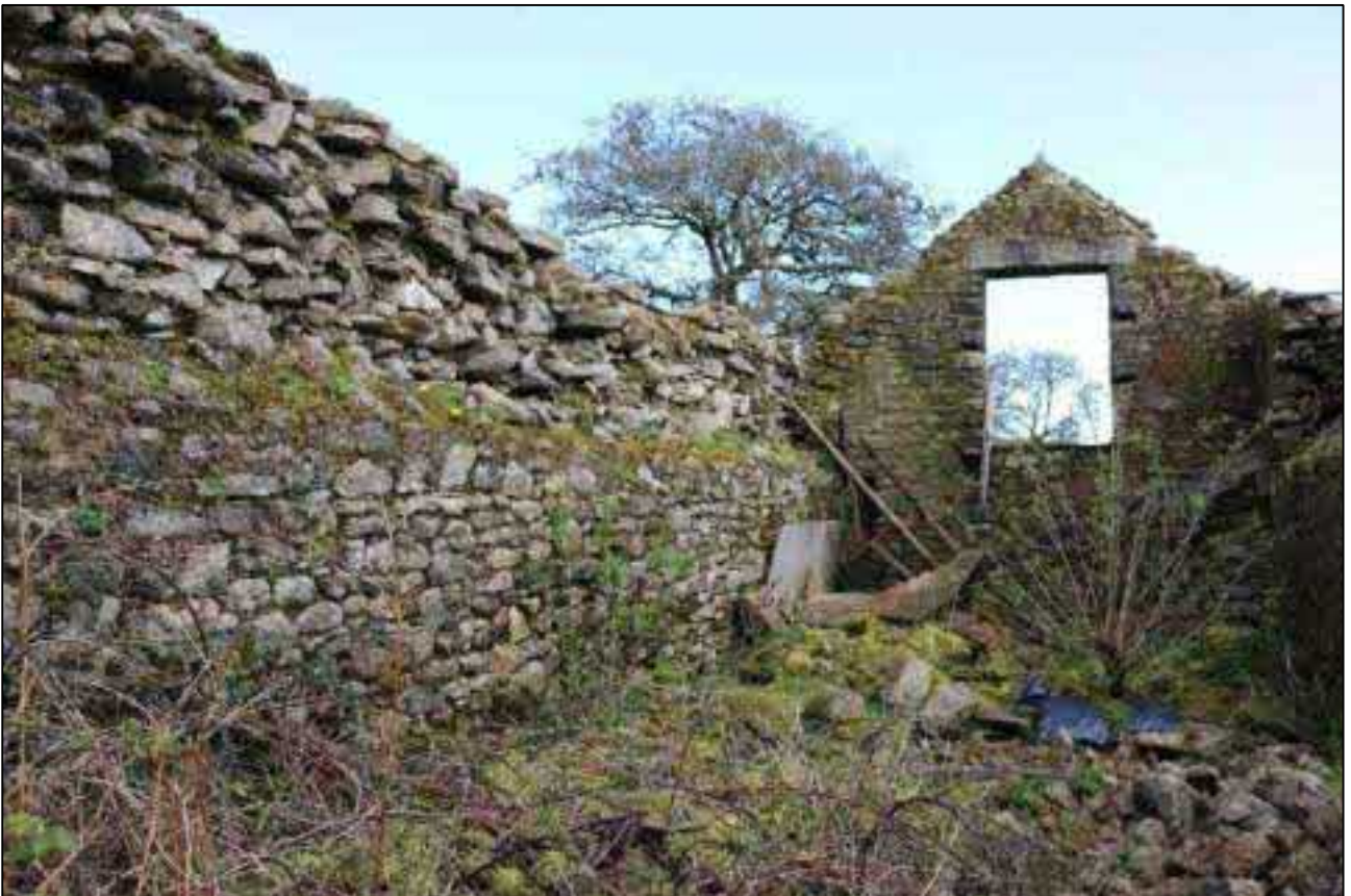
32. THE INTERNAL WEST ELEVATION LEADING TO NORTH GABLE END B1A; VIEWED FROM THE SOUTH.
