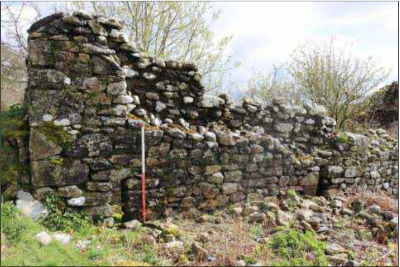
11. GROUND LEVELS CUTTING TWO GF SLITS TO SOUTH B1A; VIEWED FROM THE SOUTH (SCALE 1M).
