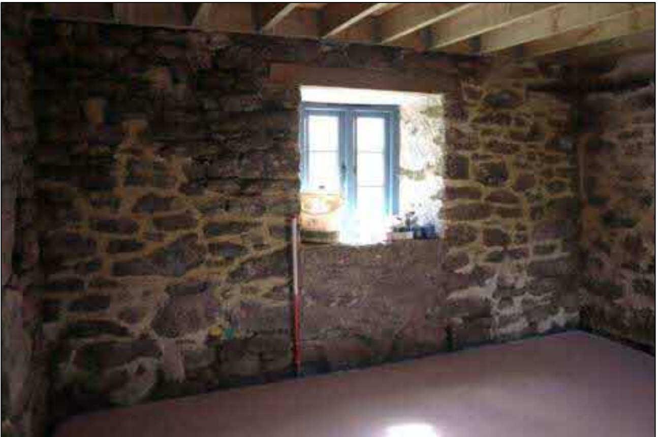
50. THE WINDOW IN A FORMER DOORWAY IN THE NORTH ROOM; VIEWED FROM THE NORTH-WEST (SCALE 1M).
