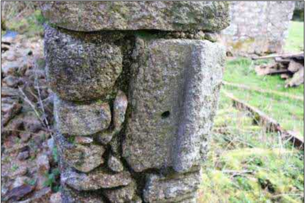
FIGURE 24: THE QUOIN WITH PROJECTING LIP AND SOCKET HOLE TO D3; VIEWED FROM THE SOUTH-WEST.
