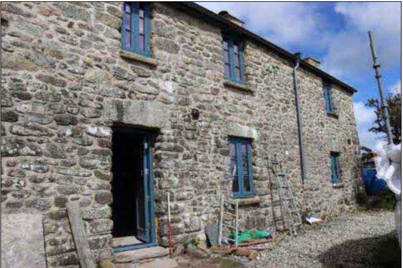
40. THE NORTH SIDE OF THE EAST ELEVATION, REPOINTING OBSCURES PHASING; VIEWED FROM THE SOUTH-EAST (SCALE 1M).
