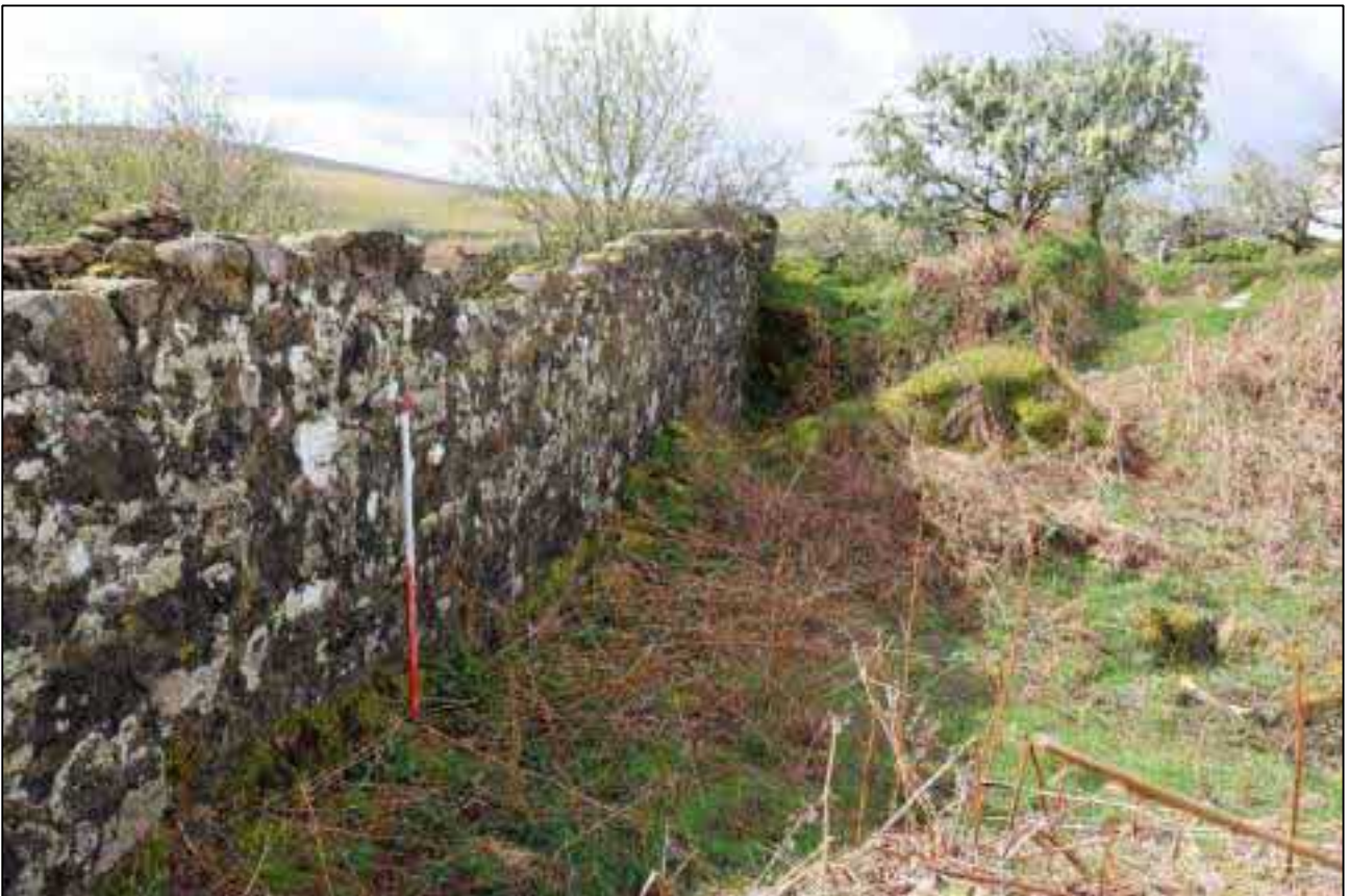
14. THE WEST ELEVATION SHOWS NO SIGNS OF AN OPENING LINKING IT TO THE HORSE WHIM; VIEWED FROM THE NORTH-EAST (SCALE 1M).
