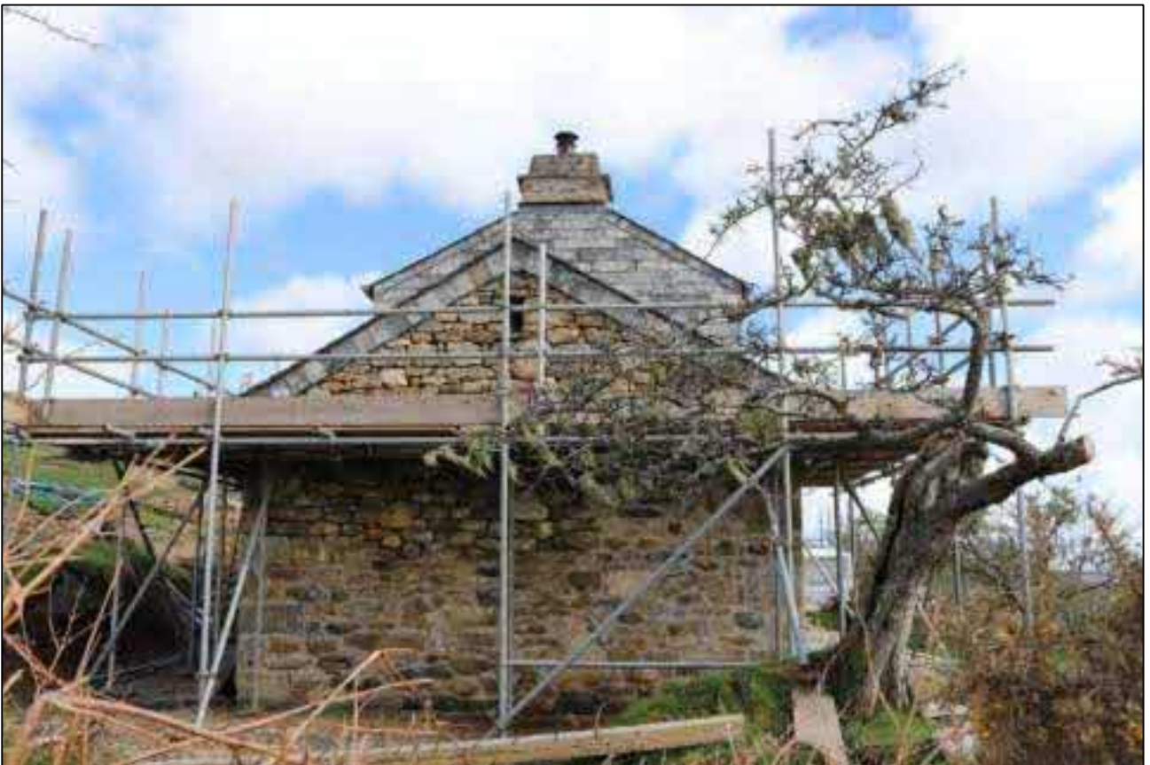
48. THE SOUTH EXTENSION, AND SLATE HANGING (MODERN) TO SOUTH WALL; VIEWED FROM THE SOUTH.
