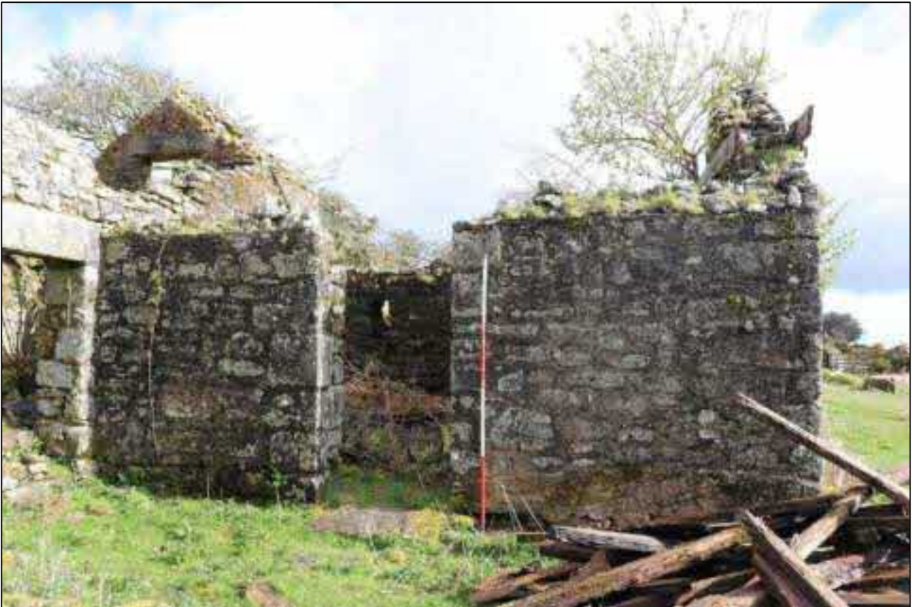
3. D5 LEADING TO B1C WITH DRESSED QUOIN DETAILS; NO LINTEL OR FITTINGS SURVIVED APART FROM THE CARVED LIP; VIEWED FROM THE SOUTH-EAST (SCALE 2M).
