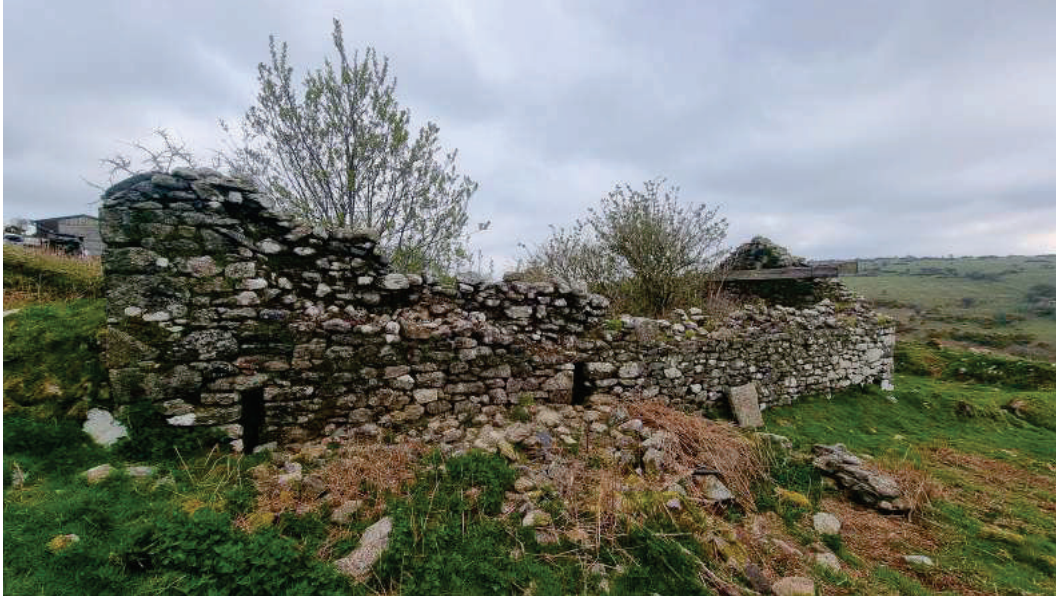
Photograph 5.0 - Outward collapsed masonry near south western quoin
