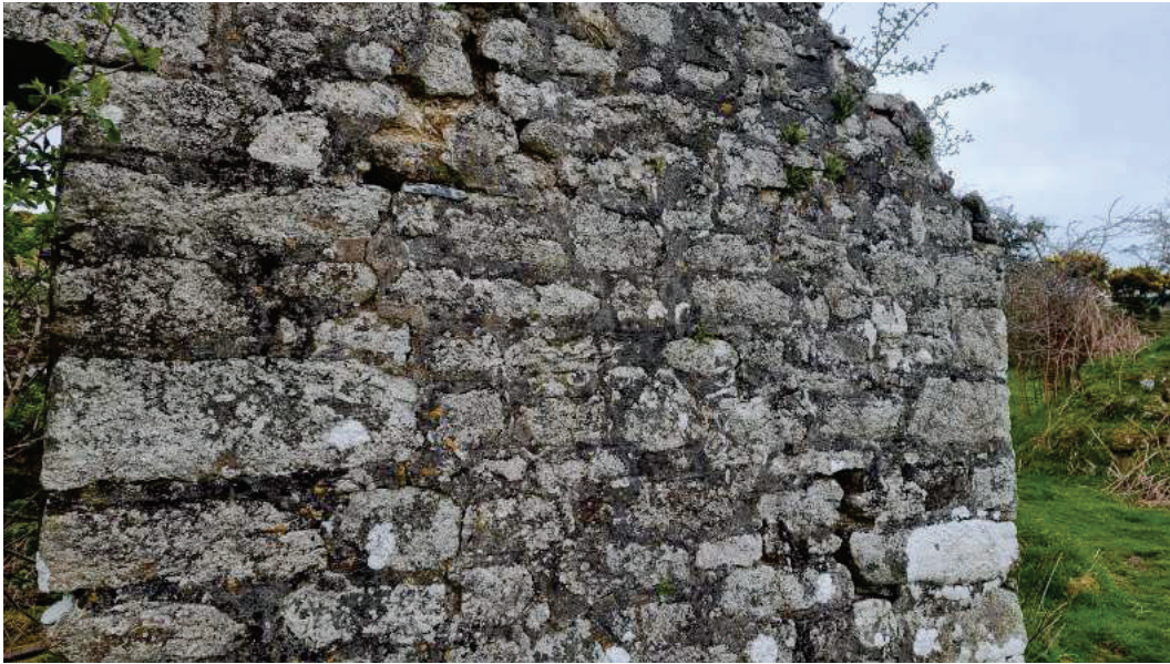
Photograph 10.0 - Vertical cracking to front elevation gable wall
