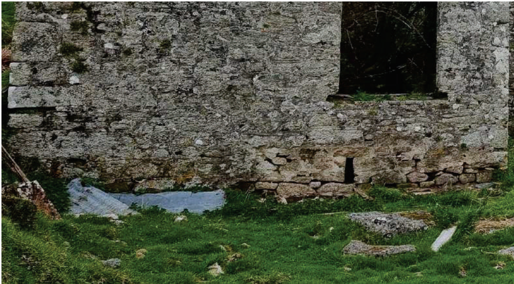
Photograph 7.0 – Voids to base of wall at front elevation
