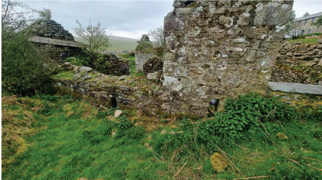
Photograph 9.0 - Build up of ground to external face with original levels unclear
