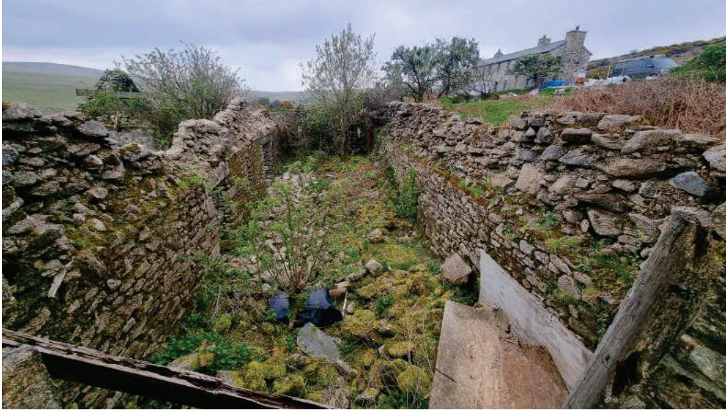
Photograph 3.0 – De-lamination of masonry to flank walls
