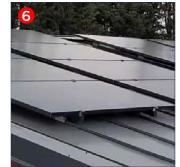
6 Solar Photovoltaic Panels Manufacturer: JA Solar 12 Years Guarantee
