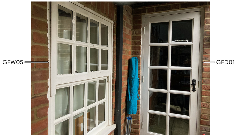
Fig.4 Photograph of Ground Floor side openings labelled (see window and door schedule for more information 114.LBC.003)
