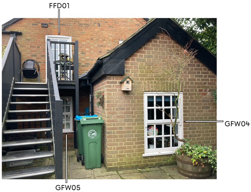
Fig.3 Photograph of Side Elevation with openings labelled (see window and door schedule for more information 114.LBC.003)
