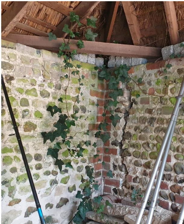
Interior view – showing crack on western wall
