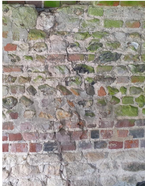
Interior view – showing crack on southern wall
