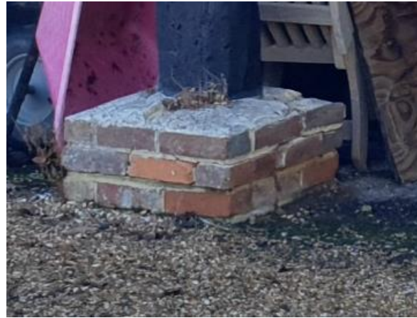
Brick plinth to timber post in need of repair
