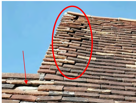
Figure 75. Example of missing and lifted roof tiles
