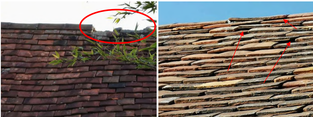
Figure 76. Missing ridge tile and lifted roof tiles
