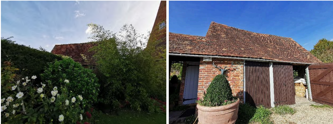
Figure 71. View of the western (left) and eastern (right) elevations of the garage
