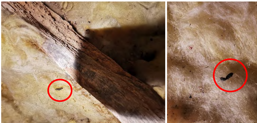
Figure 70. Bat droppings found in the loft space
