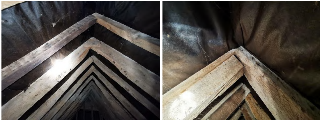
Figure 69. No ridge beam present
