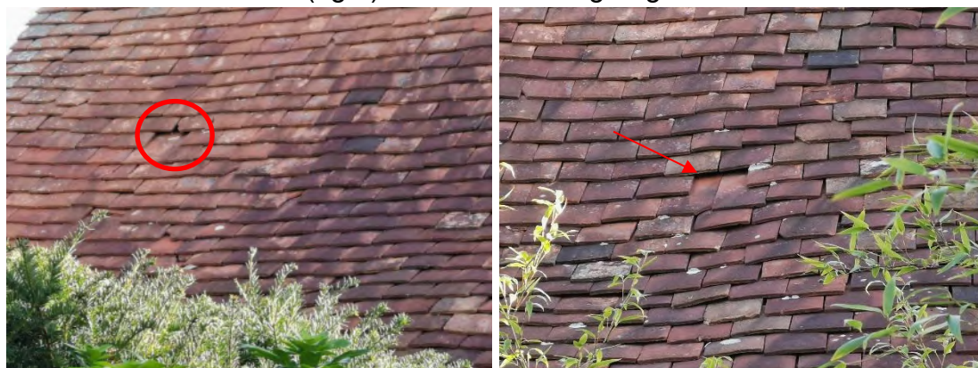
Figure 73. Example of missing and lifted roof tiles
