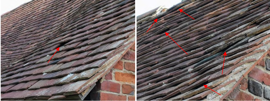
Figure 74. Example of missing and lifted roof tiles
