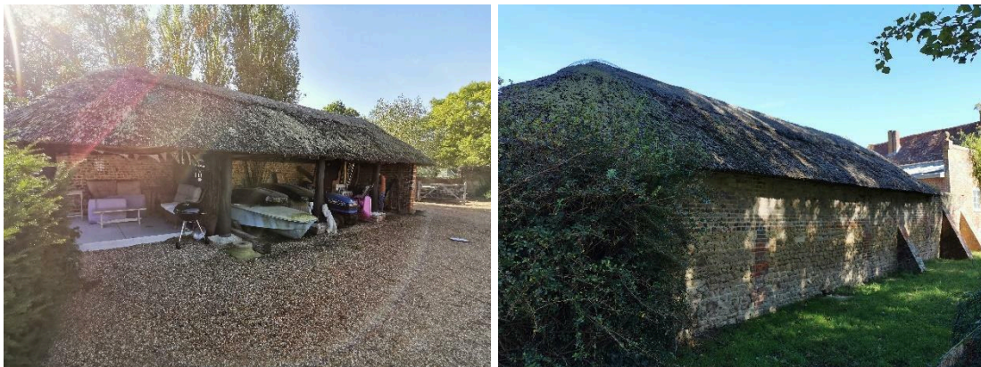
Figure 83. View of the southern (right) and northern elevations (right) of the thatched carport
