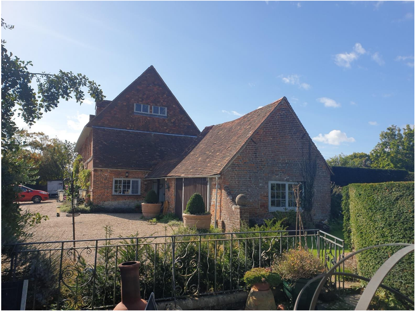
Fig 3 East elevation (note major crack over window & brick alterations)
