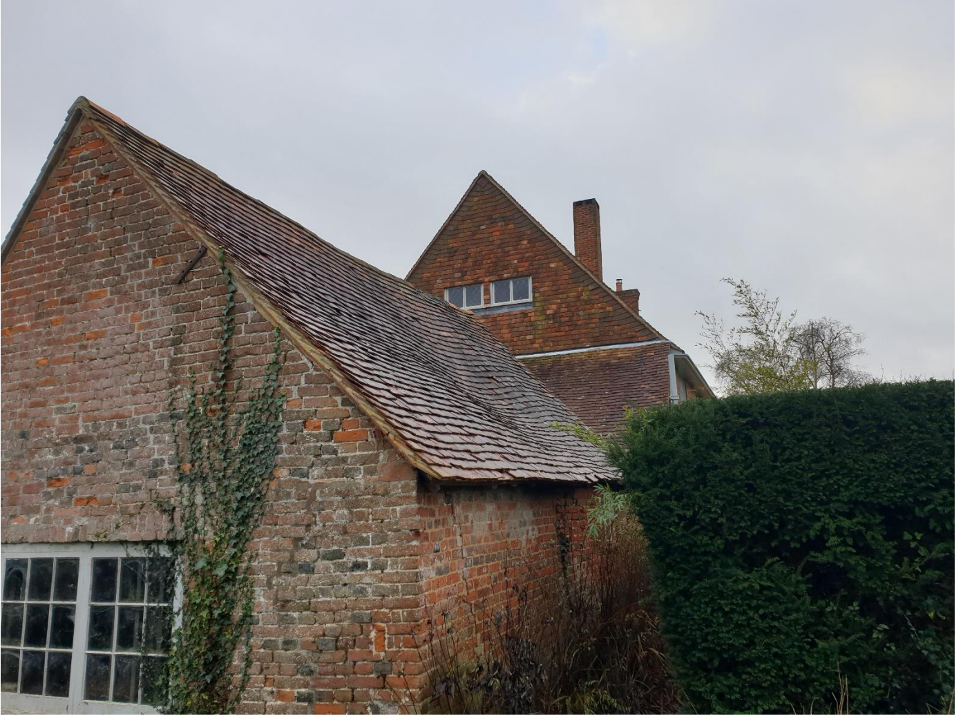
Fig 4 Garage roof failure
