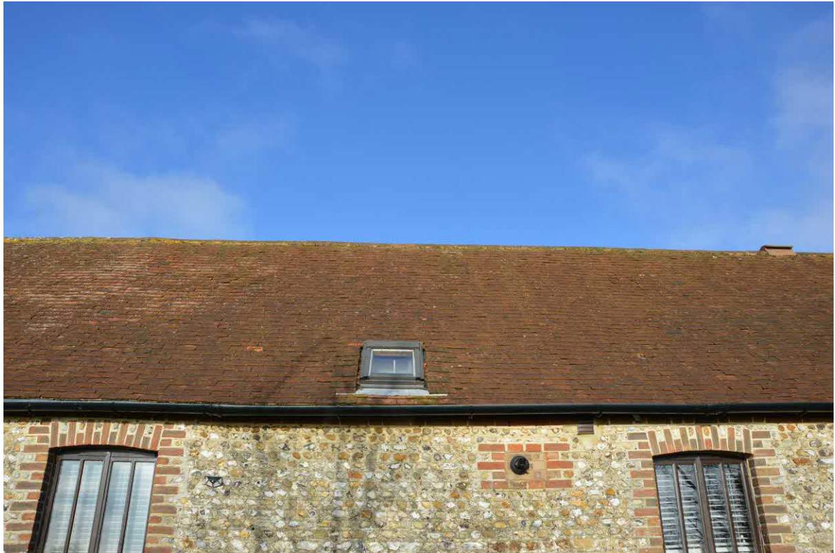
Plate 3. The south elevation of the house where a skylight will be installed.
