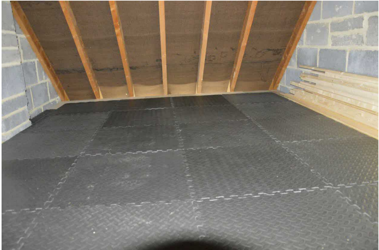
Plate 7. The roof space of the main garage where a skylight will be fitted.
