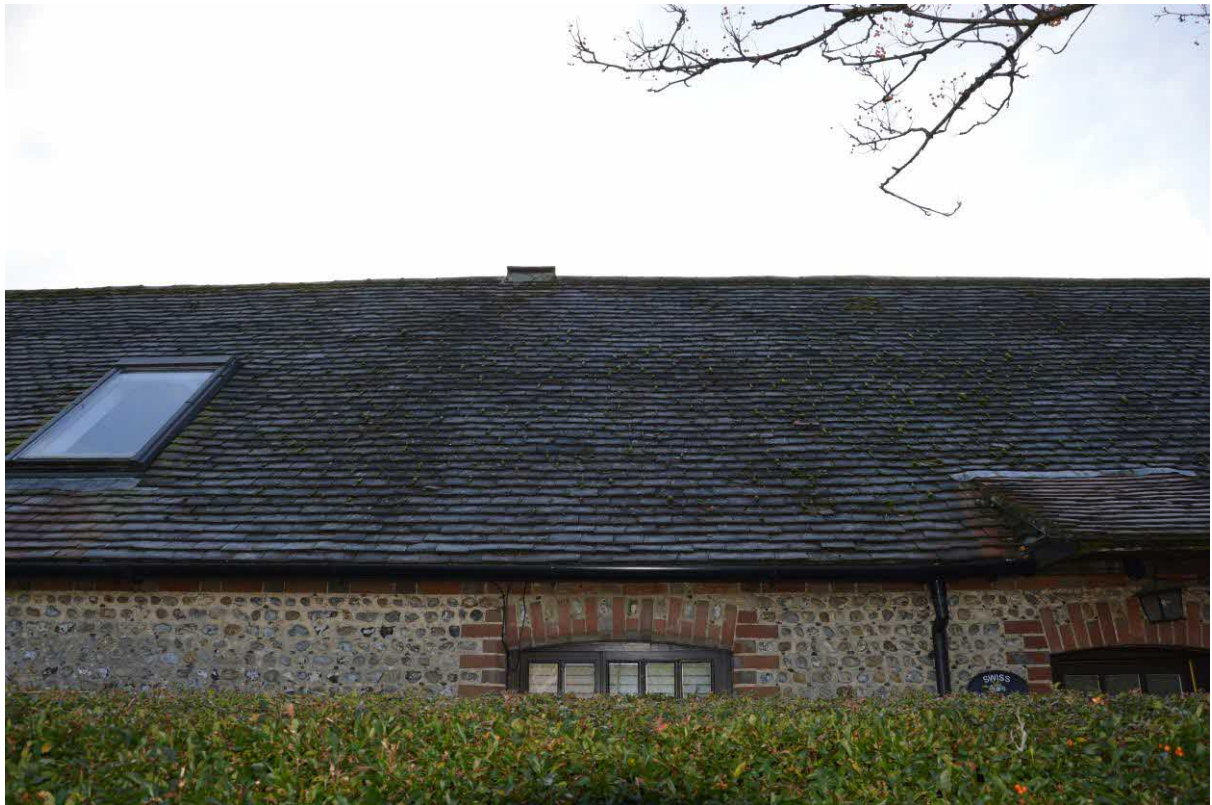
Plate 1. The north elevation of the house where a skylight will be installed.
