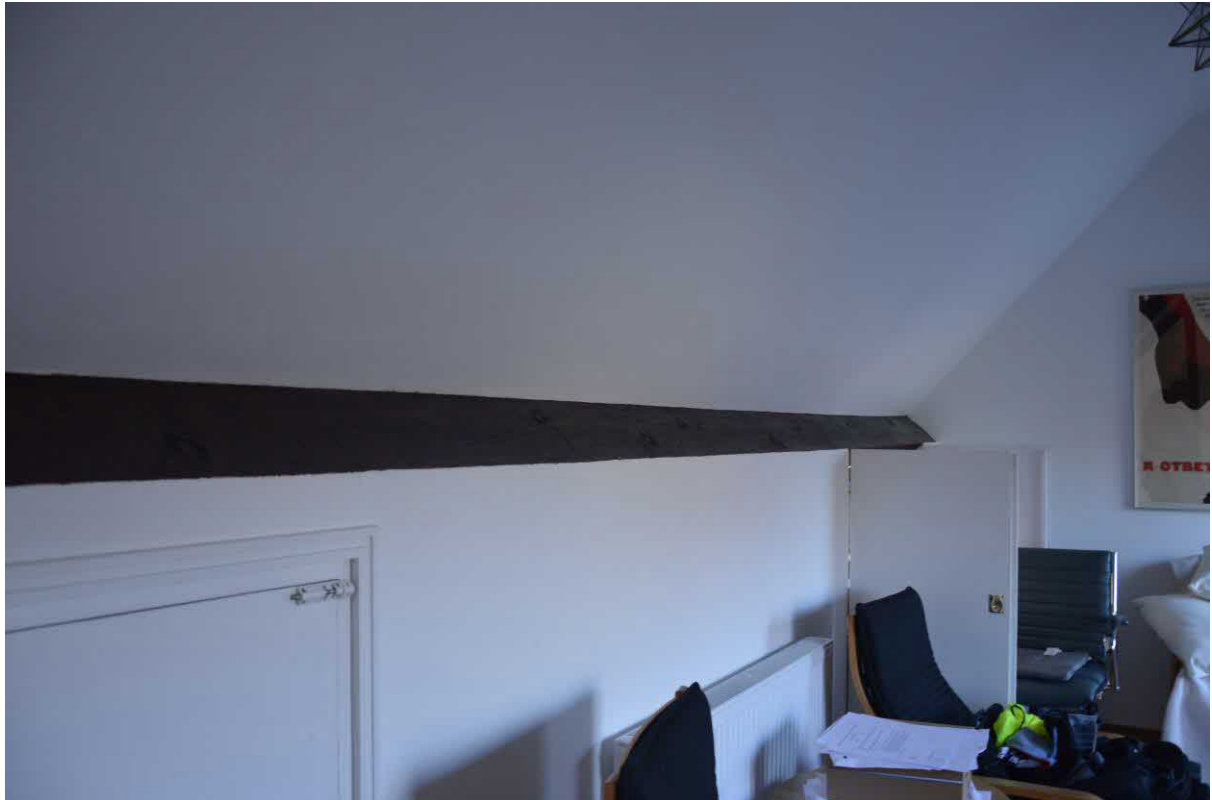
Plate 5. The internal south elevation of the house where a skylight will be installed.
