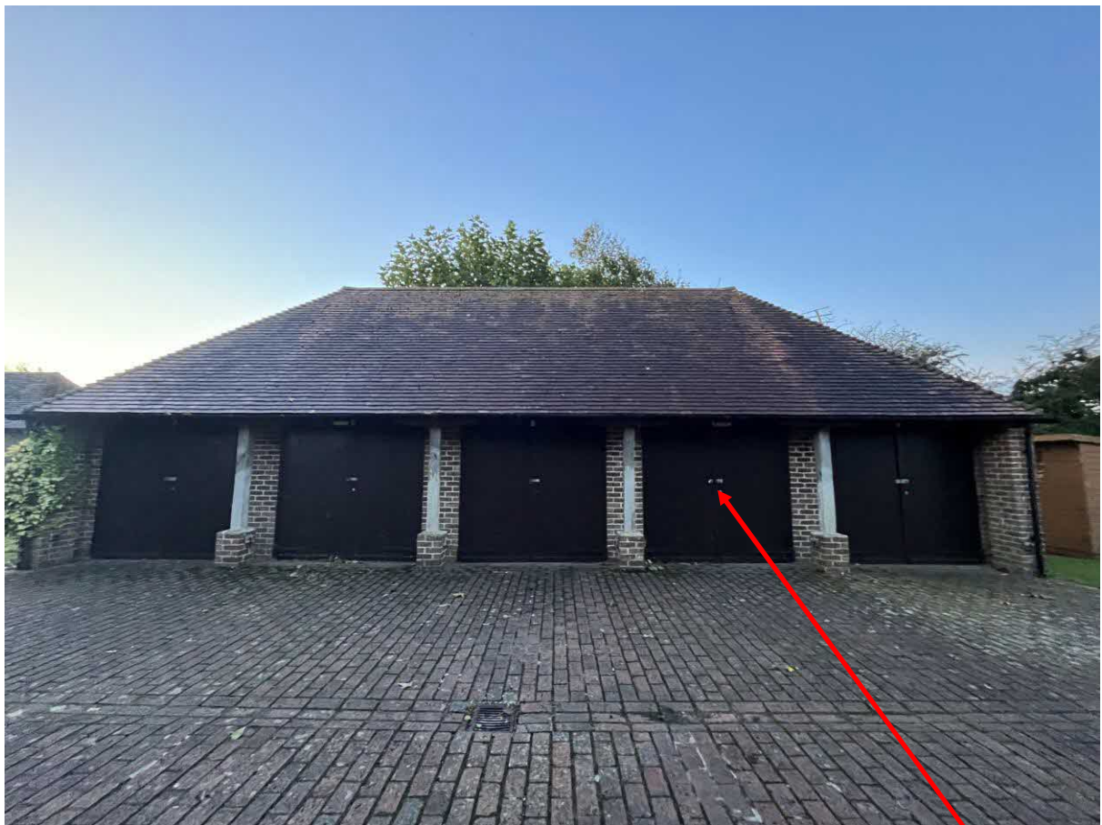
Plate 6. The block of garages showing the garage where the skylight will be fitted.
