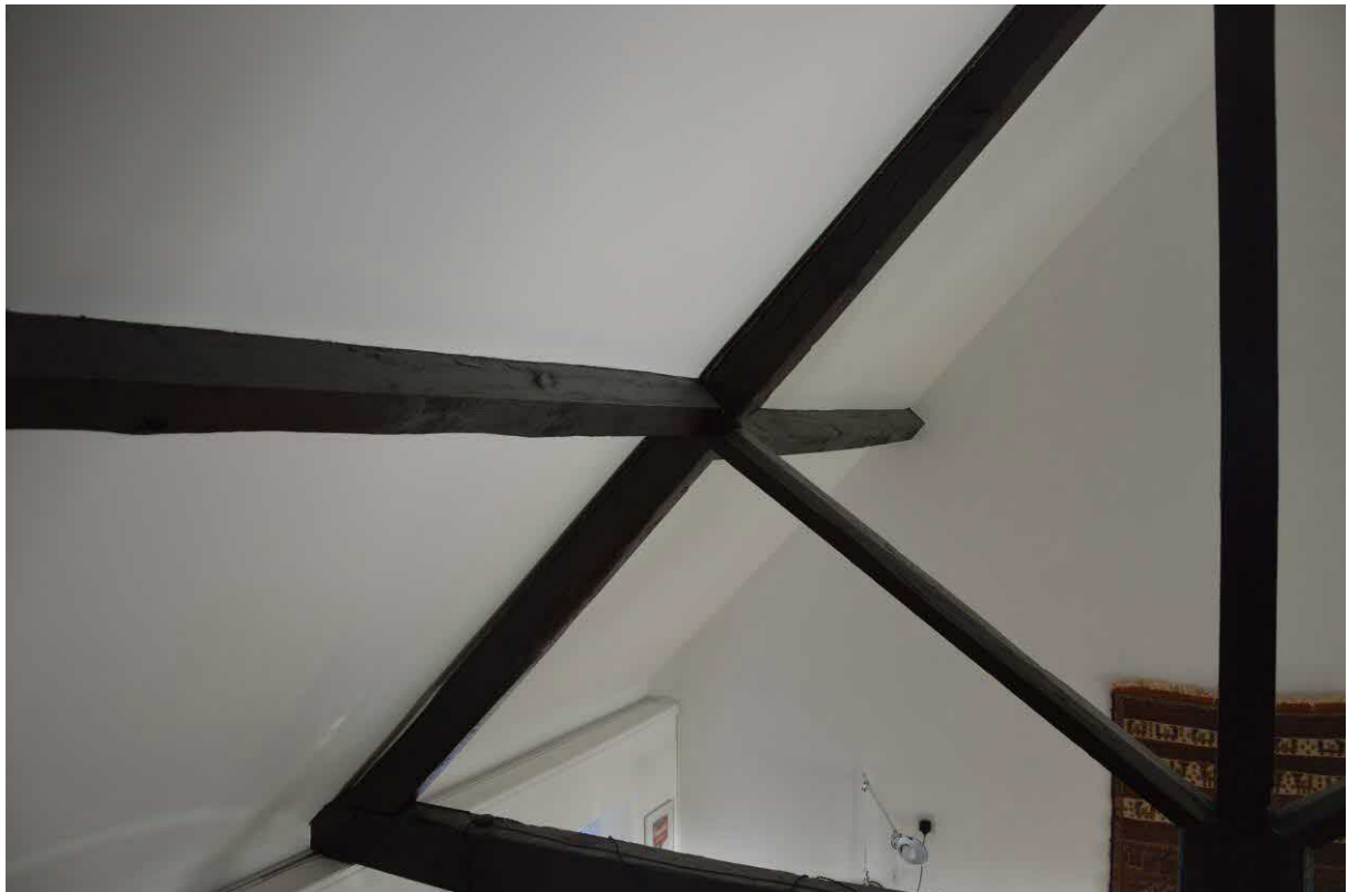
Plate 4. The internal north elevation of the house where a skylight will be installed.
