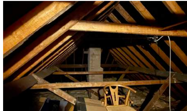
Low roof attic space - inappropriate as habitable space
