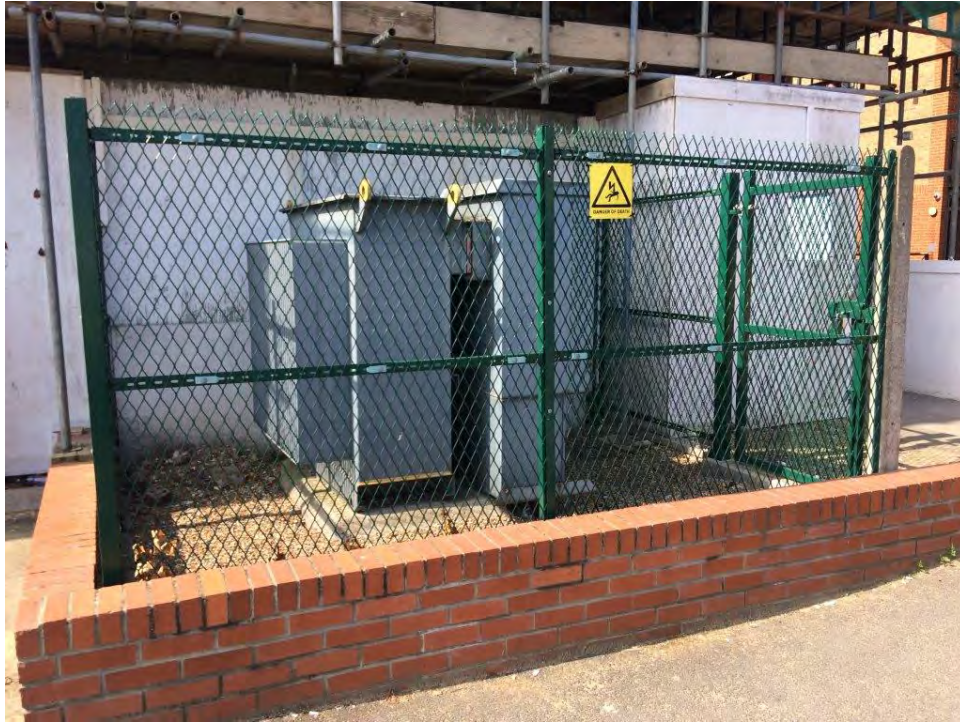
Photograph 5: The electricity substation located in the southwest corner of the carpark
