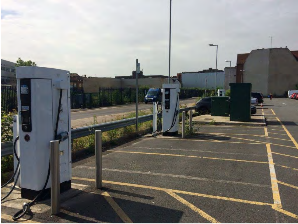
Photograph 7: Electric-car charging infrastructure
