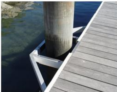
Example of a Pylon
