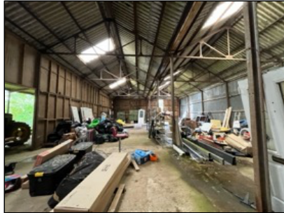
Photograph 9. Inside the barn with large sky lights provided a large amount of daylight.
