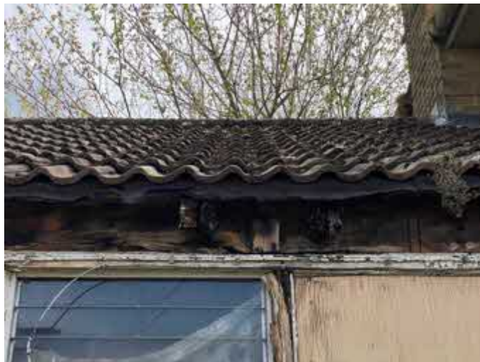
Photograph 12: Missing fascia board and soffit providing direct access into the single storey section interior.
