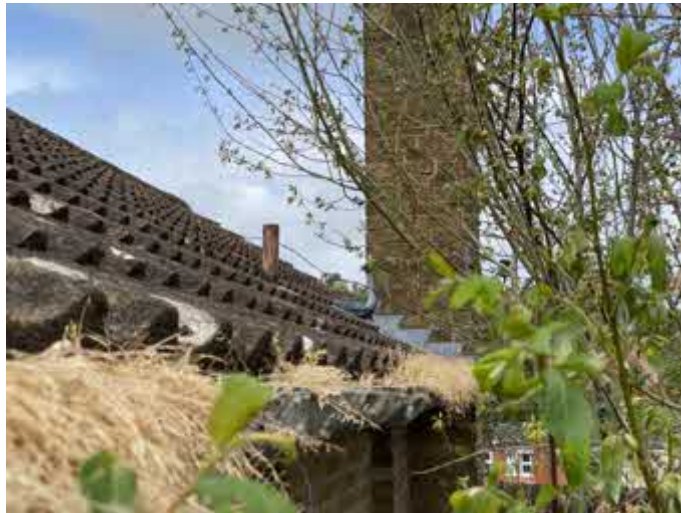
Photograph 11: Tight fitting tiles. Minor gap under the flashing – no evidence of use.
